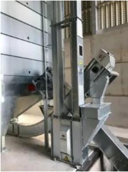
Skandia Elevator handling equipment installed with Svegma continuous now grain drier.
