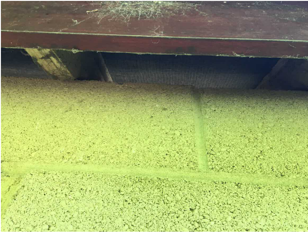
Photograph 3 –Gap between roof and northern wall of stables
