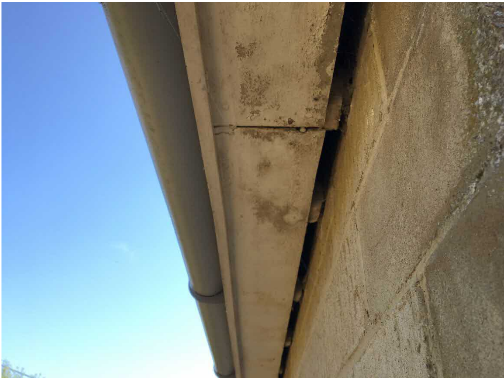
Photograph 6 –Gap behind soffit on bungalow
