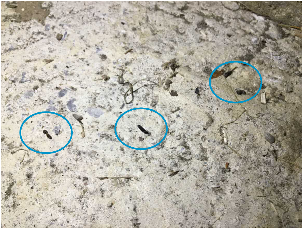
Photograph 7 –Droppings found within the stables
