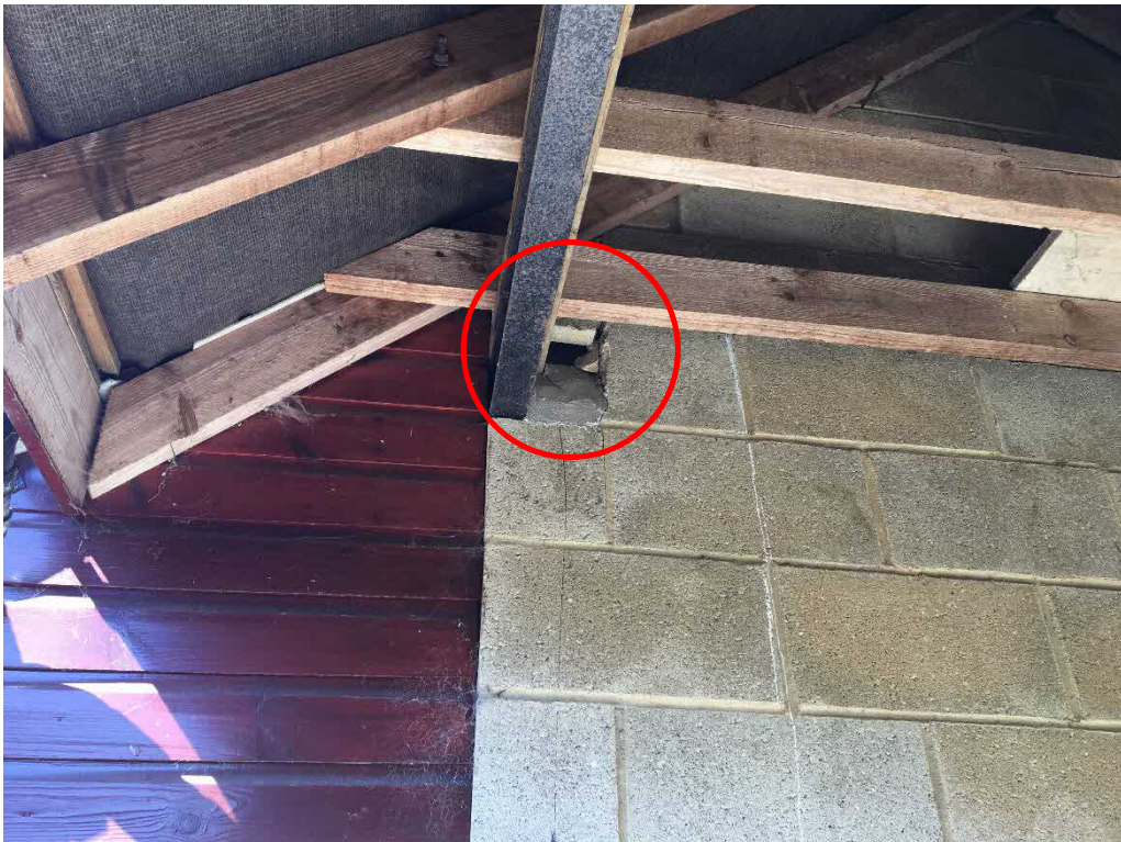
Photograph 4 –Hole in western wall of south-facing open-fronted section at east end of stables, allowing access into interior of stables
