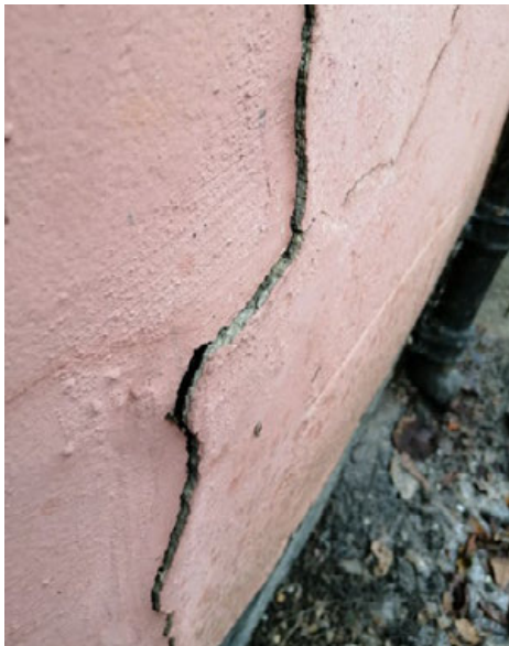
Detail of cracked render on east side of former butcher's shop
