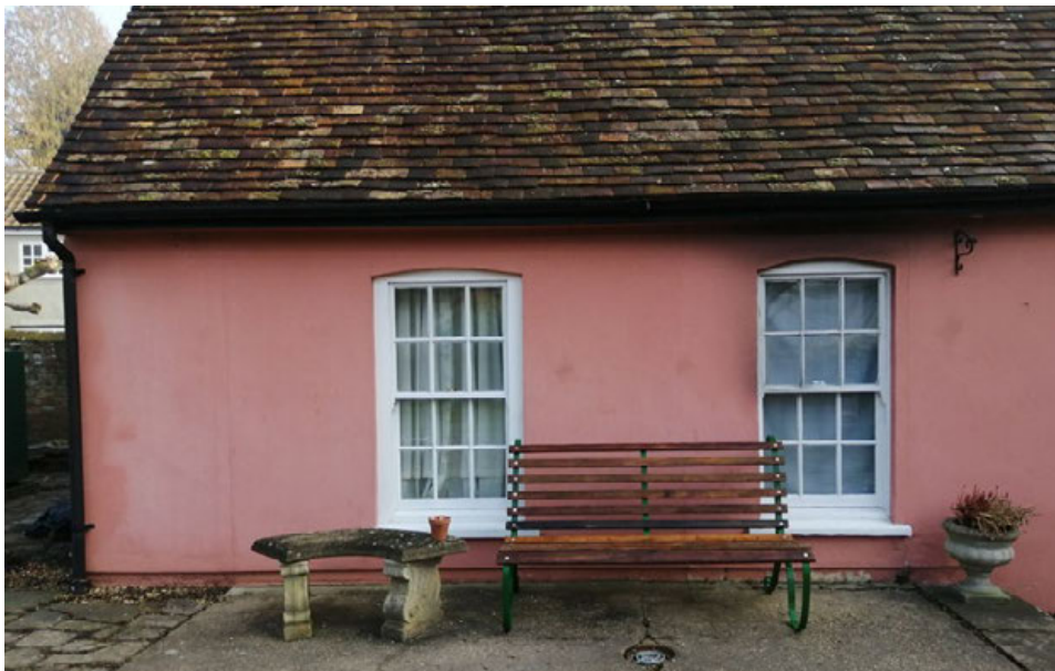
West elevation of northern range showing the former garage opening in the northern end. The location of the former garage opening is discernable by render cracks between the corner and left-side window and just to the right of the right-side window. The redundant lintel is also visible just below eaves level.
