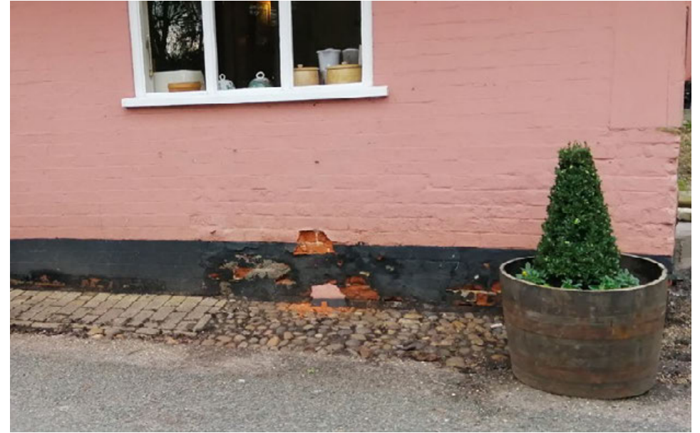
Deteriorating brickwork at low level of former butcher's shop needing repair/replacement and redecoration
