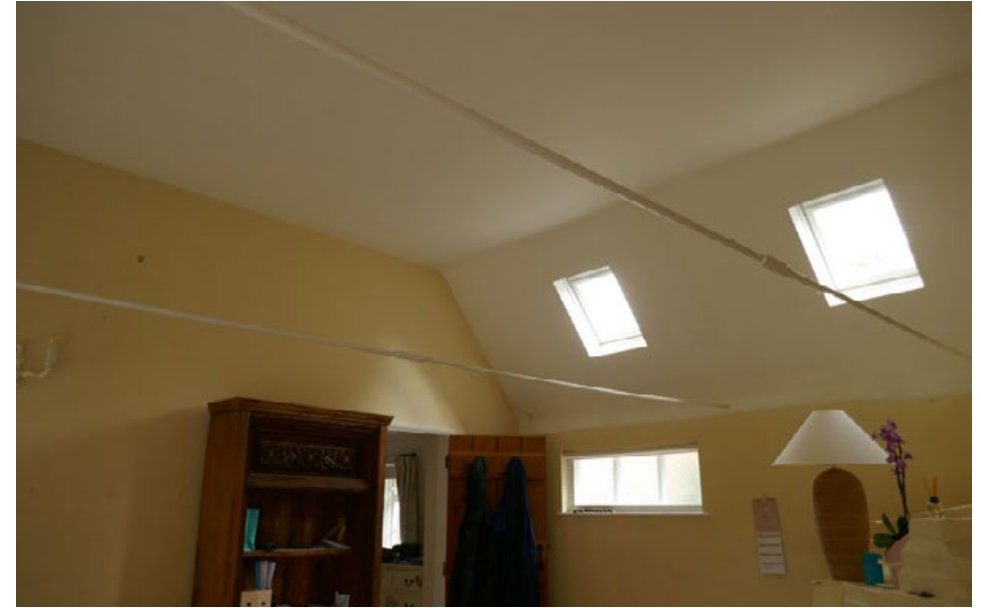
11 Kitchen - Steel tie bars, rooflights, ceiling, and blockwork partition wall (left hand side) to be removed. A queen post truss is to be installed in place of the blockwork partition wall.
