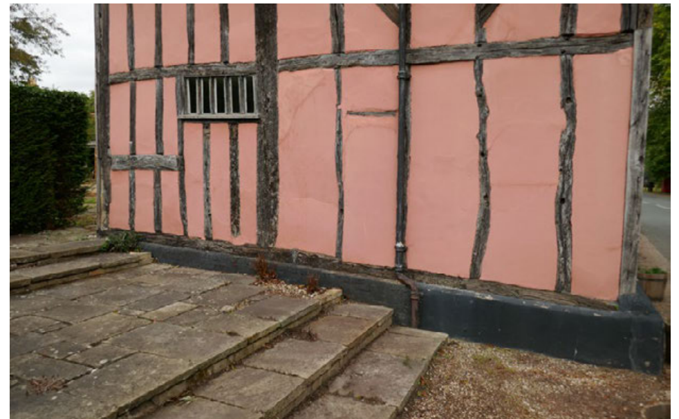
Concrete steps to the west elevation where it is proposed to replace with a low-level brick retaining wall and evergreen hedge
