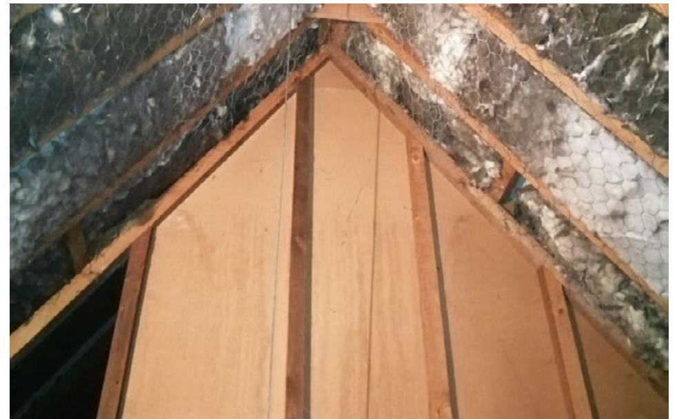
23 & 24 Stair & Bedroom 4 - View of 21st century partition wall and roof structure on north side of proposed new stair and Bedroom 4
