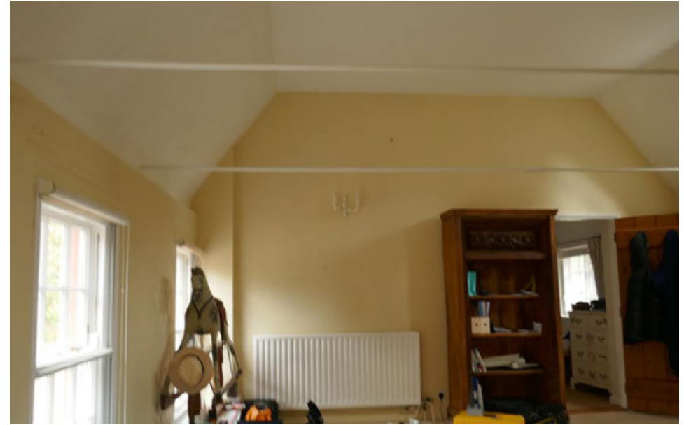
Interior of north wing, showing blockwork partition wall in location of former garage, with steel ties above.
