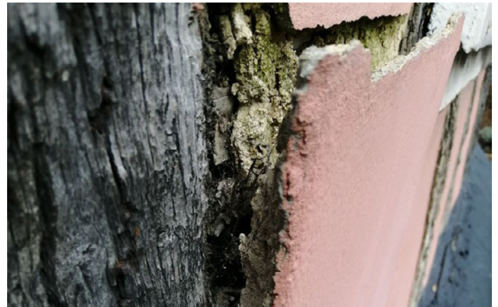
Image showing failing cement render
