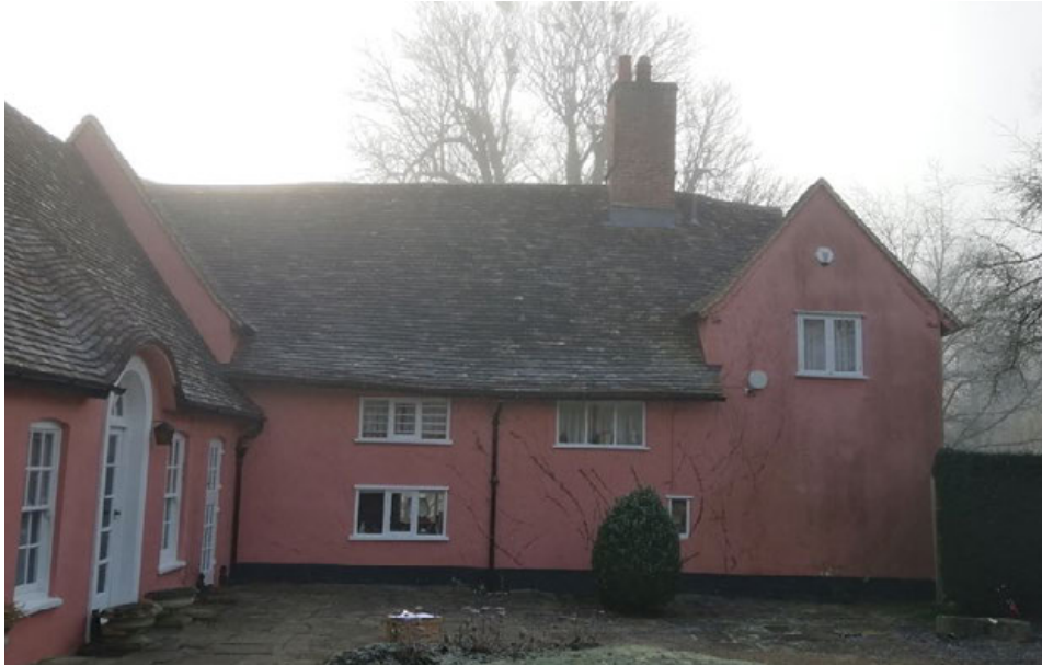
North elevation showing area of cement render to be removed and replaced with lime render
