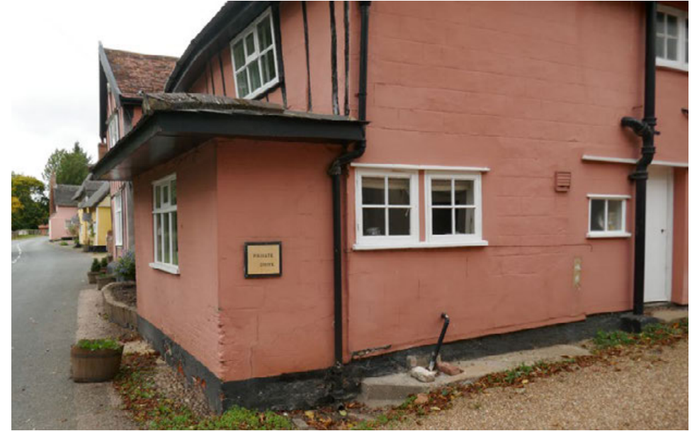
Southern end of east elevation showing deteriorating render and leaking shallow pitch roof with concrete hip tiles and eaves without gutters
