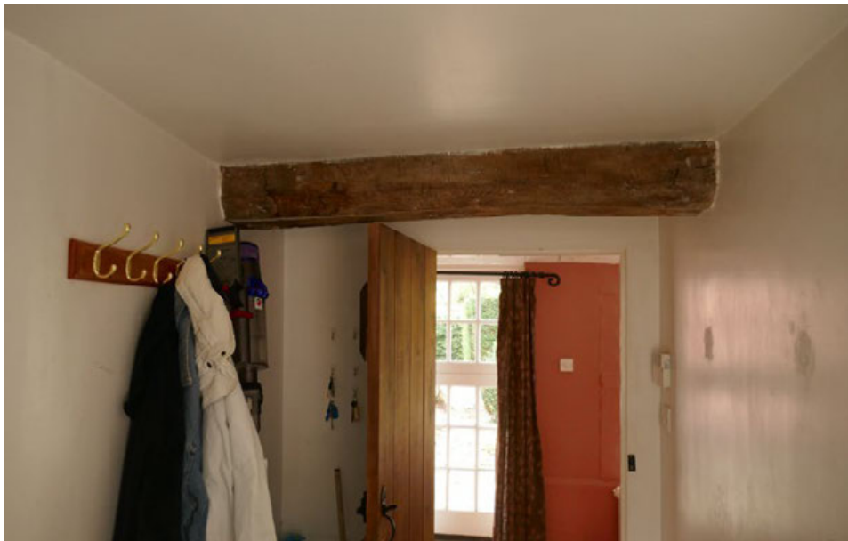
10 Utility - Existing spine beam to be retained. Plasterboard finishes and partition walls to be removed.
