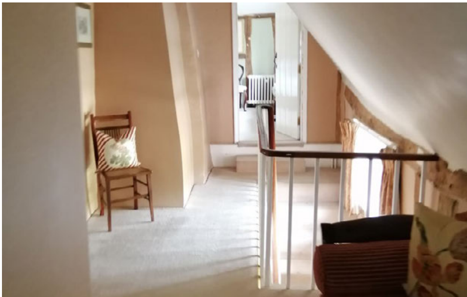
16 Bedroom Lobby - Area of proposed Bedroom Lobby showing awkward head height and unsafe landing in front of bedroom, along with late 20th century balusters and handrail to be removed
