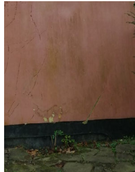
Detail of cracked render on north elevation
