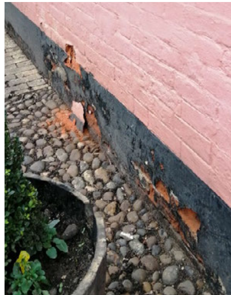
Detail of deteriorating brickwork in need of repair on south side of former butcher's shop
