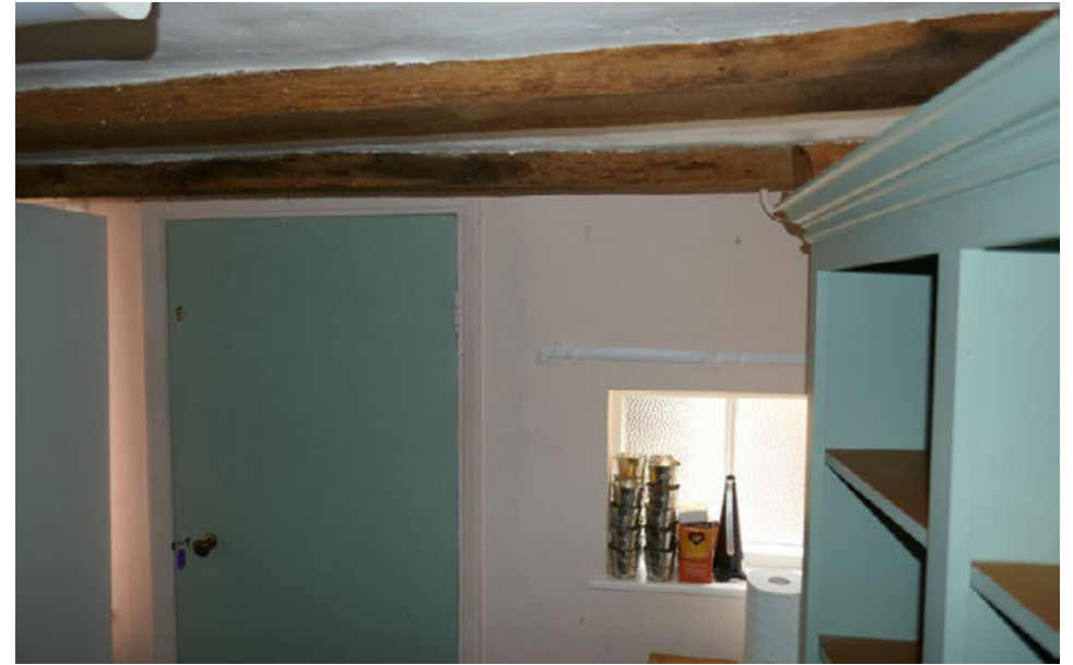
7 WC & Boots- External door and window to be replaced in adjusted window opening
