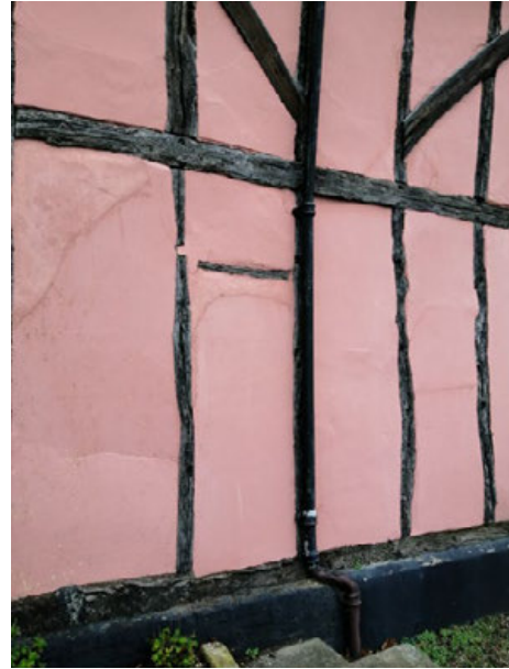
Existing rainwater pipe on western elevation to be altered and plinth to be repaired
