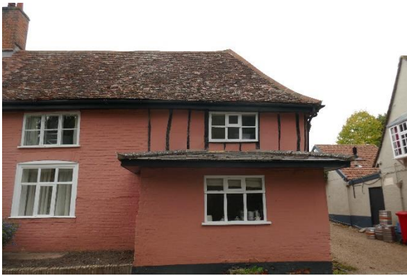
Photo 1: South eastern façade of house, with small single storey, slate tiled extension – to be re-roofed
