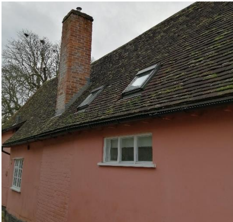
Photo 3: Roof lights on eastern façade of northern half of building – to be removed
