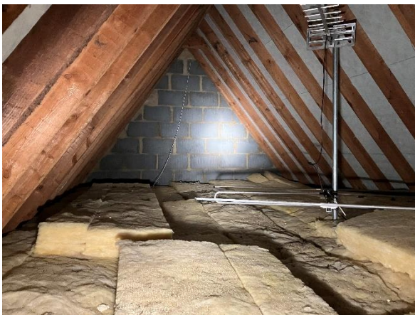
Photo 9: Internal view of central northern roof section, with new insulation laid across old bat droppings
