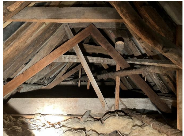
Photo 4: Roof space across southern section of the building – to remain entirely undisturbed
