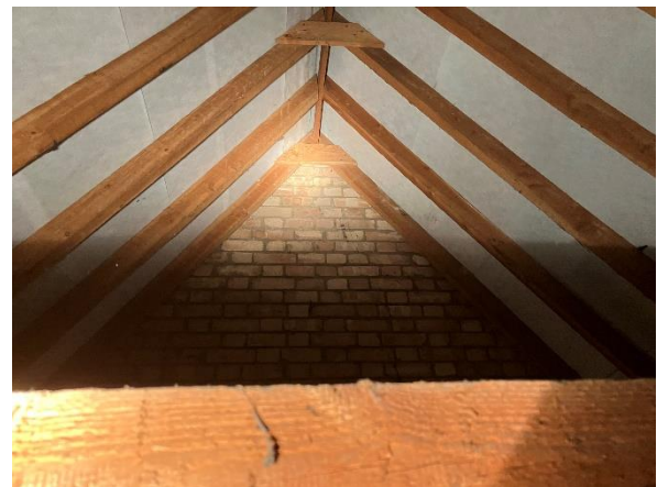
Photo 10: Northern gable wall, inside northern most loft of northern roof section. (Loft too short and tall to obtain full field of view with camera)
