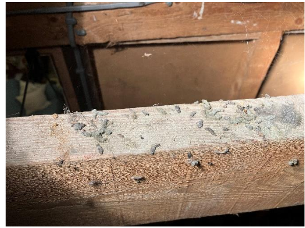
Photo 8: 30-40 dry and very dusty likely BLE droppings on an undisturbed roof beam in northern roof space
