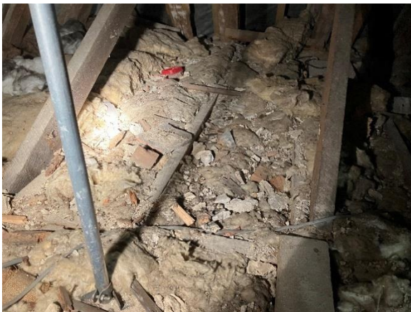
Photo 5: Lime plaster, wood offcuts, general debris and dust typical of floor space in southern loft
