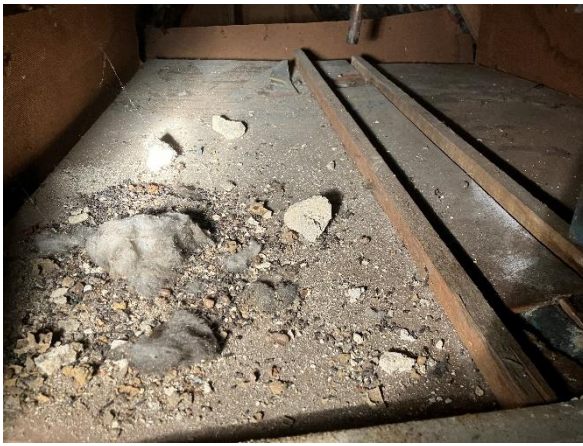
Photo 7: Collection of c.100 dry and dusty bat droppings on top of water tank cover, along with rubble and debris likely produced during re-roofing work
