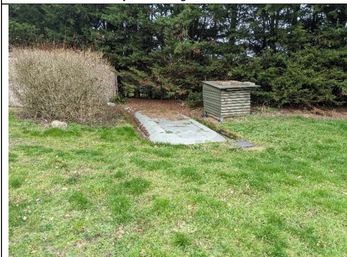
Photo 5 Sewage treatment plant to be fenced off
