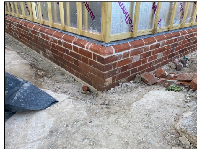
Plinth Brickwork to Front roadside elevation; Original bricks reclaimed from existing building demolition
