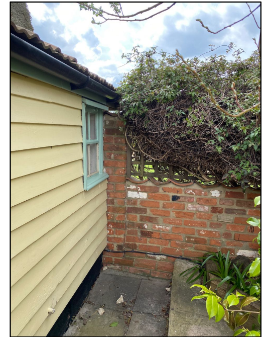
New Timber Cladding; Treated Feather Edge timber boards decorated with Dulux Weathershield County Cream to match existing
