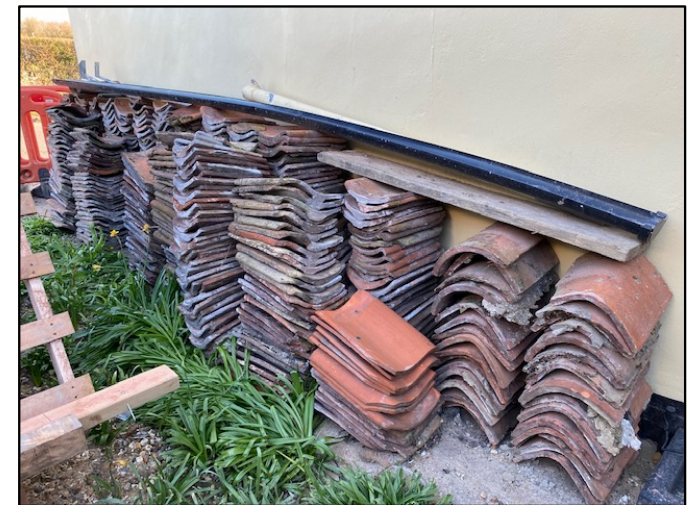
New Roof; Original clay pantiles and clay ridge reclaimed from existing building demolition. Contractor has secured additional matching tiles for any shortfall in quantity. Where existing roof extends to form intersection with new roof, roof finish to comprise newer clay pantiles to match existing.
