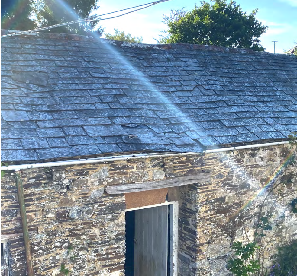
02: BARN ROOF DAMAGE DETAIL
