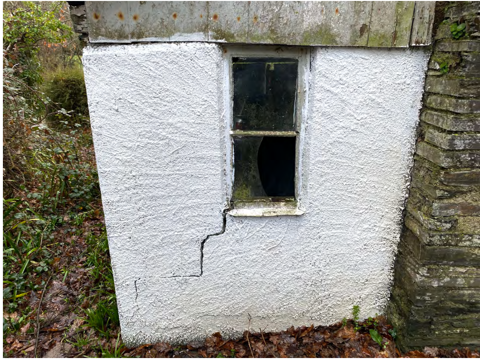
14: GARAGE NORTH ELEVATION CRACKING
