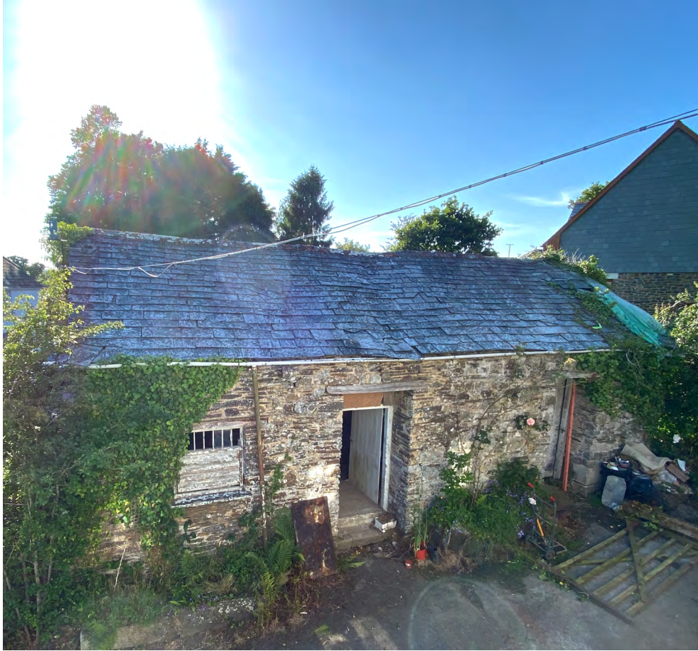
01: BARN ROOF DAMAGE
