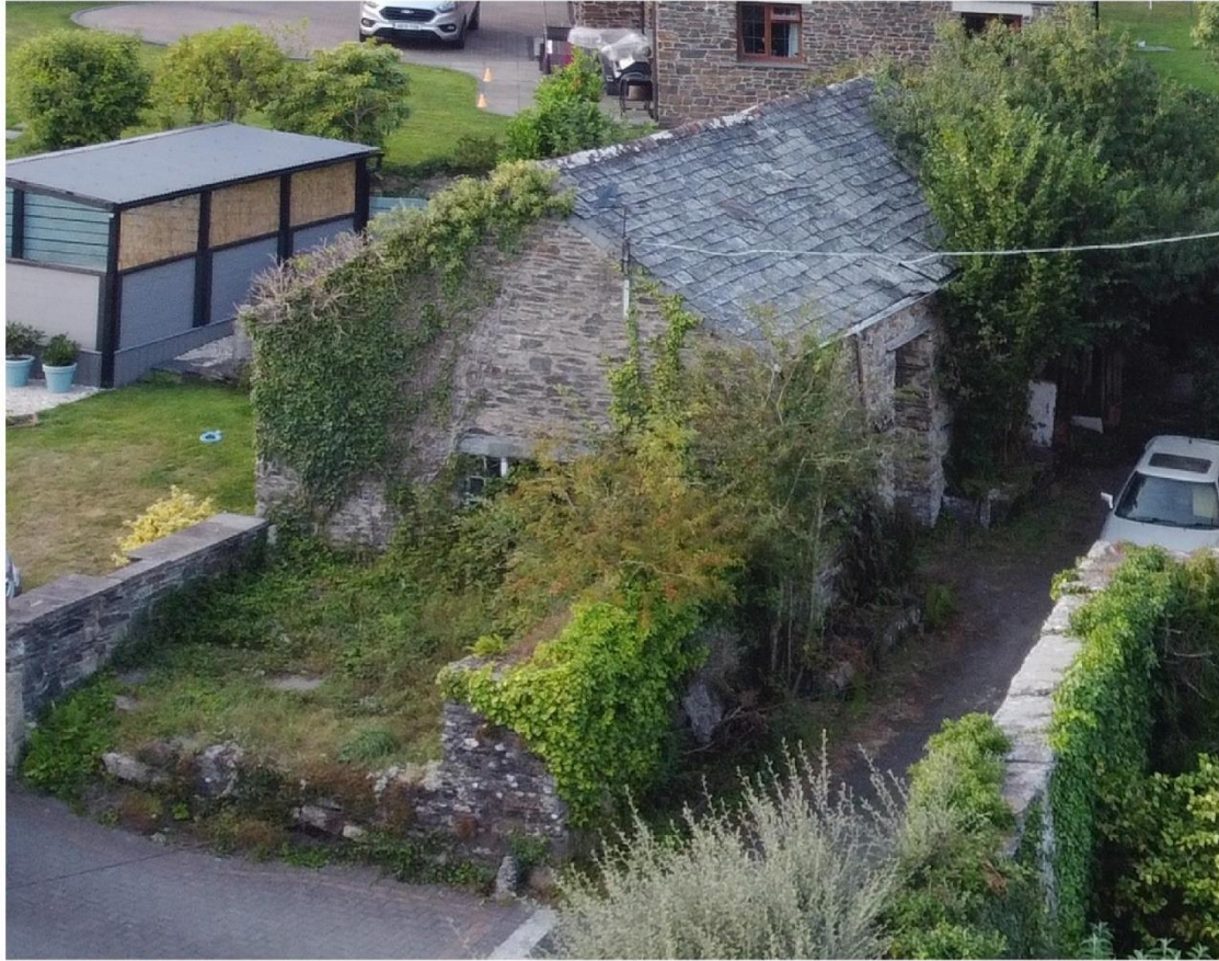
i) Outbuilding to the west of the house. Note rag slate roof and killas rubble construction
