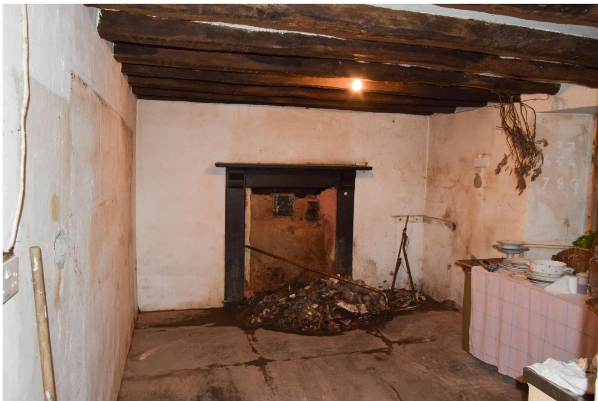
ii) Looking west across western room. Lath marks on the exposed beams evidence that this room has previously been ceiled. The fireplace is a later (c1900) insertion and has previously housed a range.
