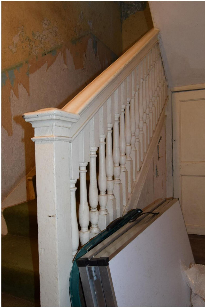
i) Principal stair (ground floor). 18th century understairs cupboard door to right
