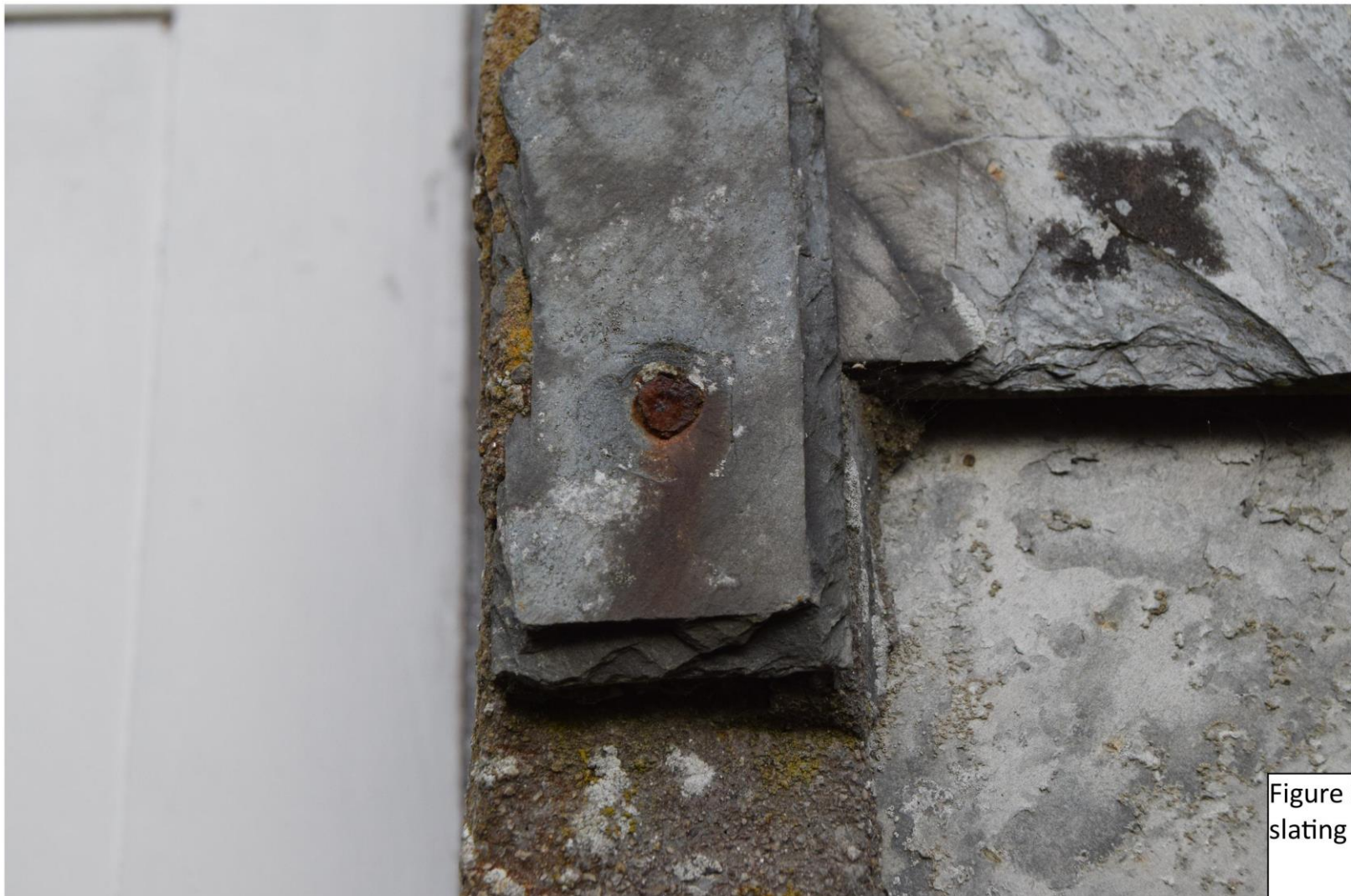
ii) Close detail of one oversealing strip showing heavily corroded screw fixing. The strip below has been failed.
