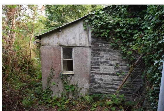
iv) the current garage, attached to the east wall of the listed front garden walls is a rendered blockwork structure with corrugated iron roof covering.
