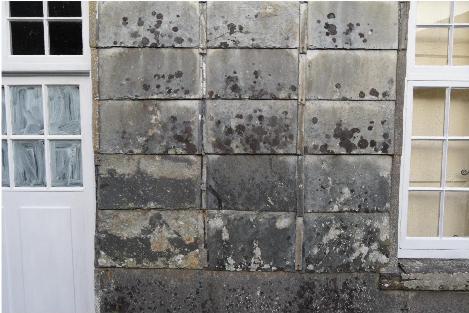
i) Detail of patent slating on the west elevation. Nove missing over sealing slates
