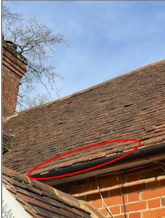
Photograph 5: Gaps under roof and ridge tiles
