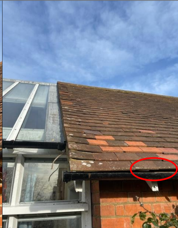
Photograph 6: Raised roof tiles.
