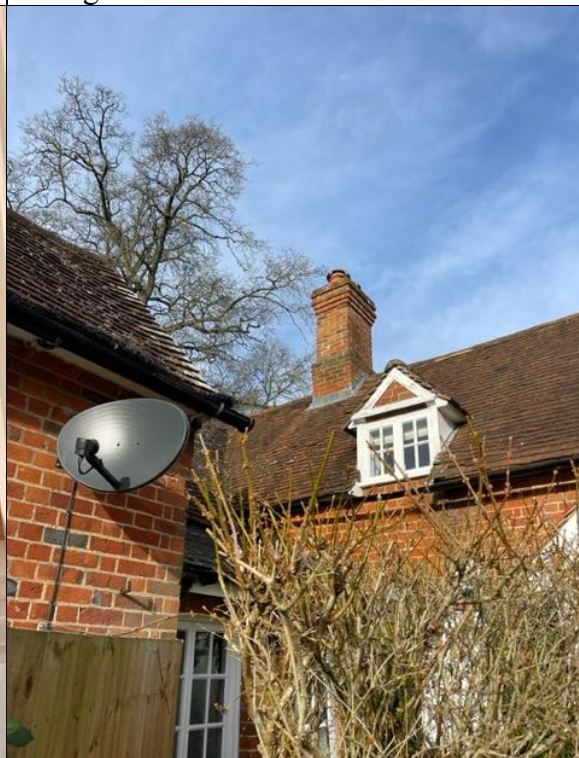
Photograph 12: Gaps under roof tiles.
