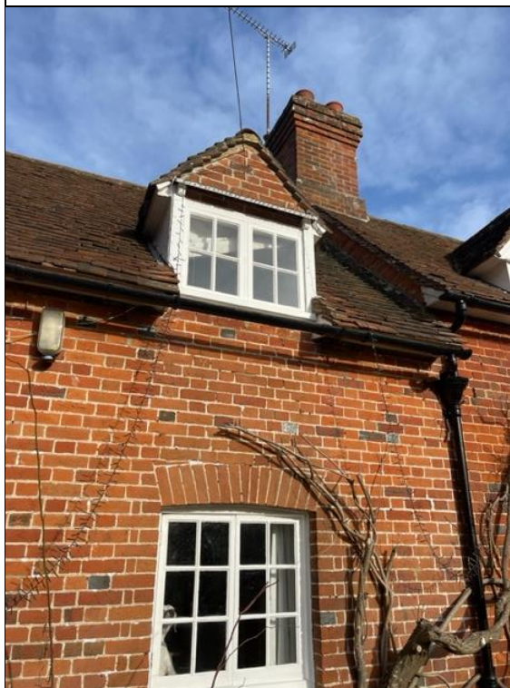
Photograph 3: Gaps under roof tiles next to dormer window.
