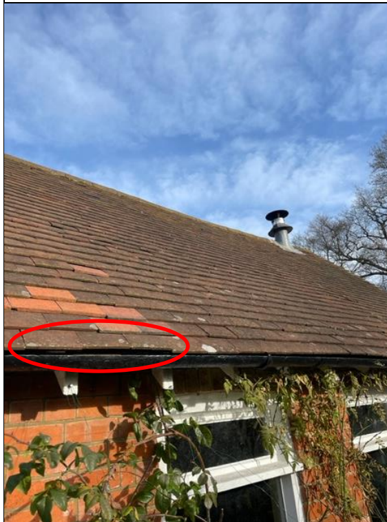
Photograph 7: Raised roof tiles.
