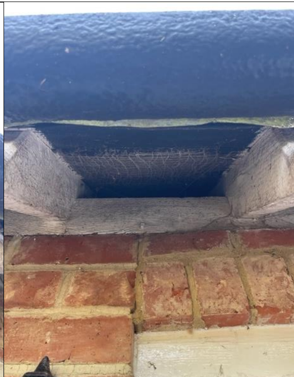
Photograph 18: Large gaps under guttering.
