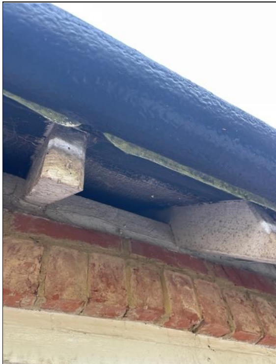
Photograph 17: Large gaps under guttering.
