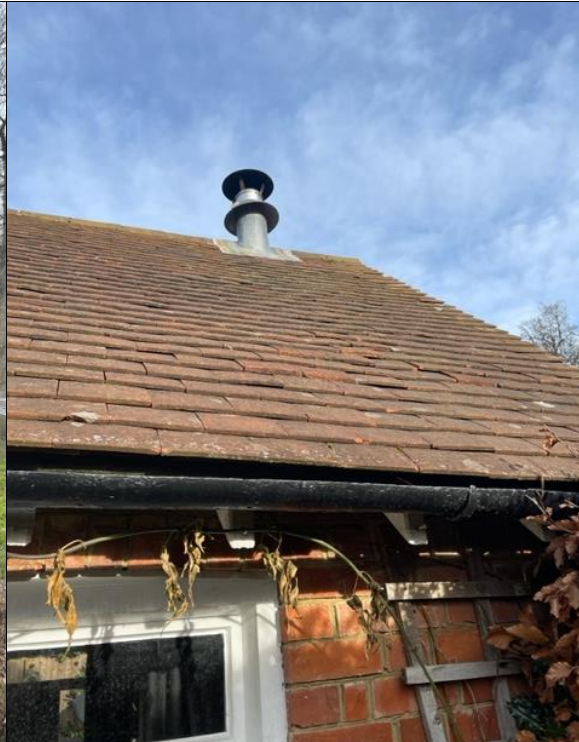
Photograph 18: Gap under guttering.
