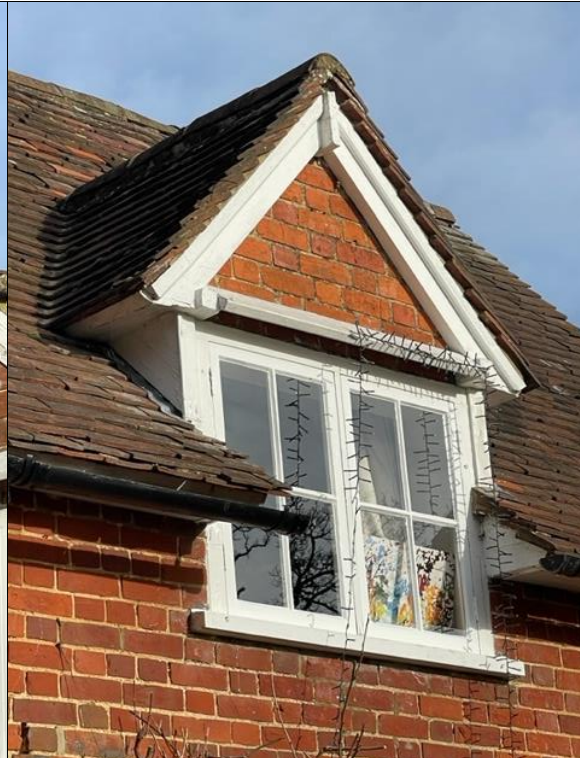
Photograph 14: Gaps under roof tiles and wooden soffits.
