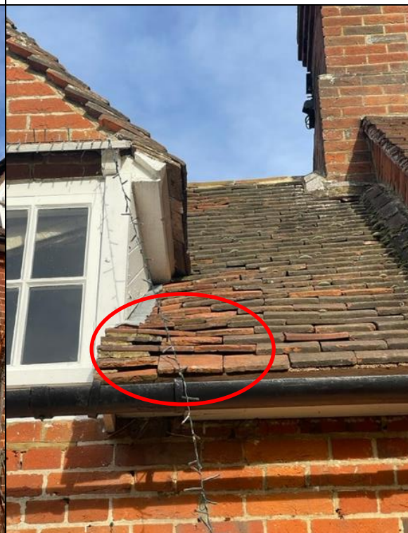
Photograph 4: Lifted tiles next to dormer window.
