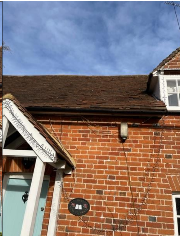
Photograph 2: Gaps under clay roof tiles.
