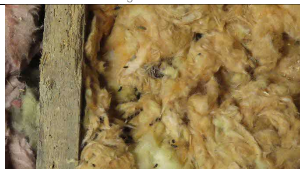
Rodent droppings in roof space
