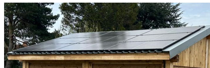
Image of solar panels
