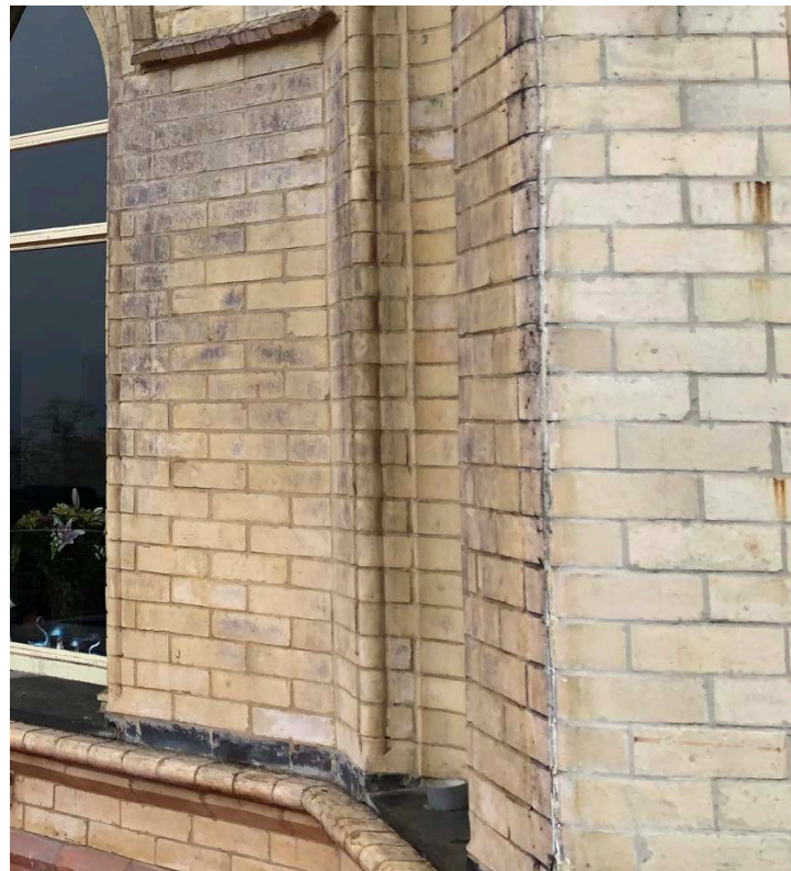
Reeve Castle. Cream-coloured Barnstaple machine-brick which includes decorative bands of red brick.
