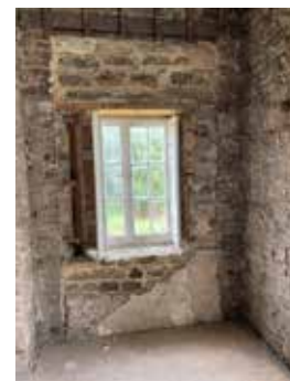
Photograph showing scarring surrounding window W36
