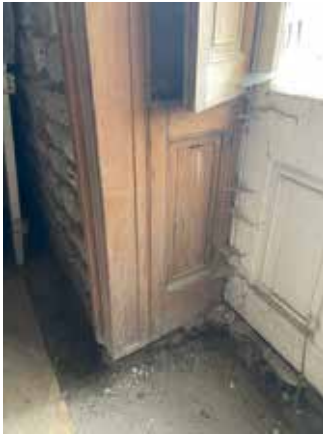
A Photograph showing the timber panelling surrounding the existing entrance door D5, which stops short of the existing floor level
