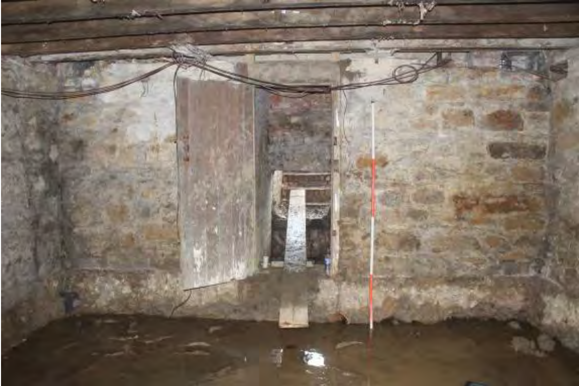
Photo 13. Door in south wall. Note substantial Victorian foundations here and drain pipe to L. of ranging rod. High level ventilation slots, top L and R
