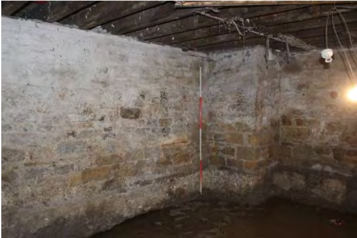
Photo 14. Pier in NW corner of cellar (providing support for large Drawing Room fireplace and associated stack). Note depth of mass concrete foundation
