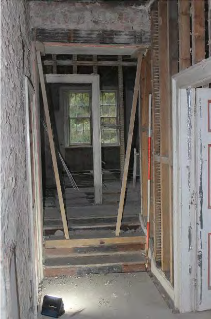
Photo 19. View looking west along landing. Wallpaper surviving behind studwork partition adjacent to ranging rod. Note timber props resting on second step and brick relieving arch over timber lintel above 1880's opening through earlier gable wall
