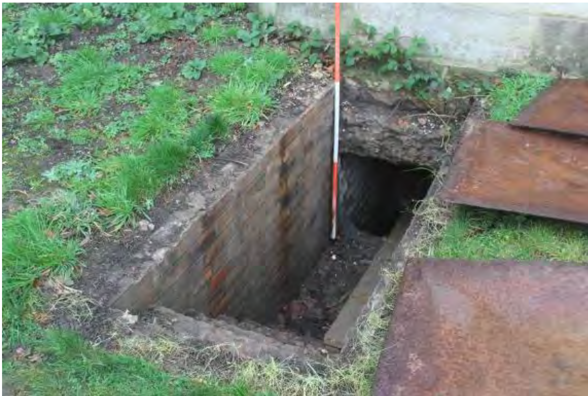
Photo 2. Steps and brick lined passage below the bay on the S. front. Note mass concrete foundation to 1880's bay and modern blocking, subsequently re-opened, behind ranging rod
