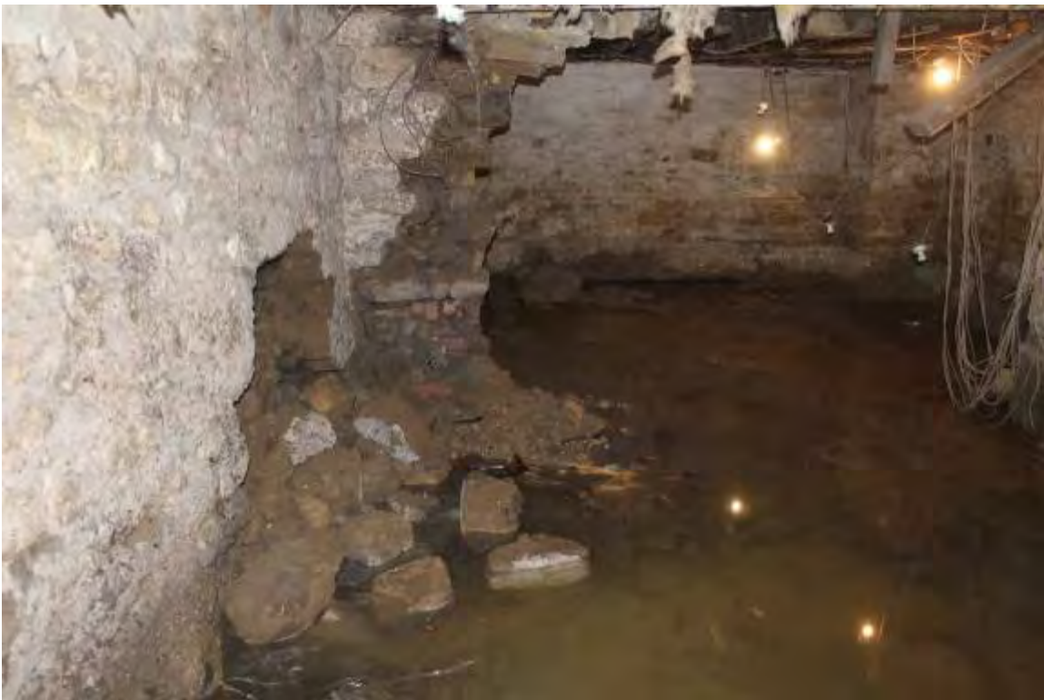
Photo 12. Stub of cross wall removed in previous works and recent collapse of unsupported south wall. 1880's cellar in background
