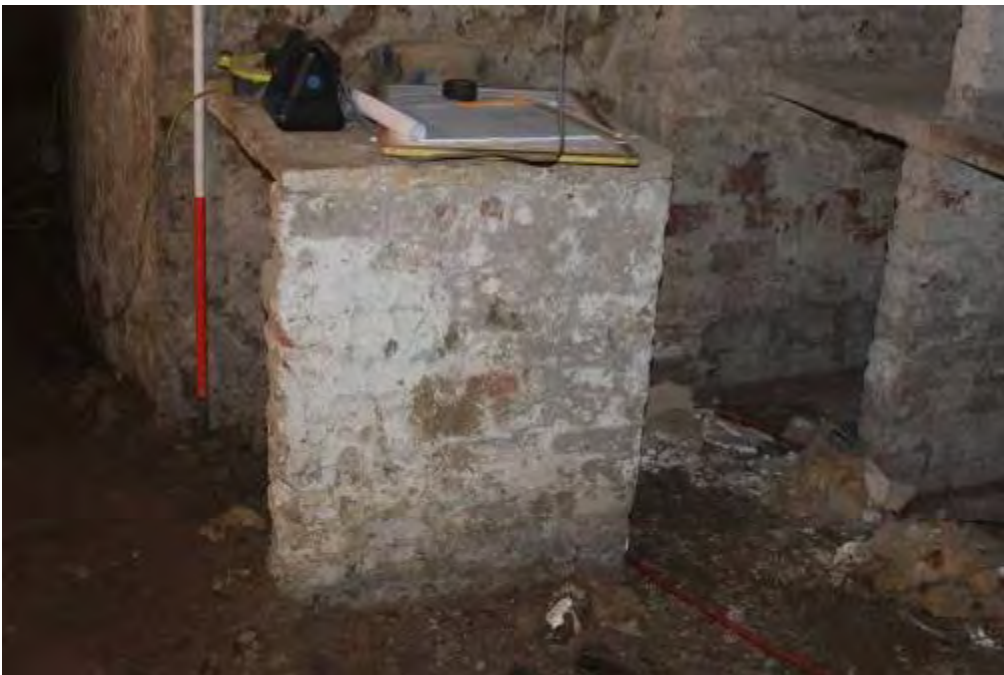
Photo 6. Stone shelf on brick pier against north wall. This would have been inside a former N/S running partition (scar visible at position of ranging rod)
