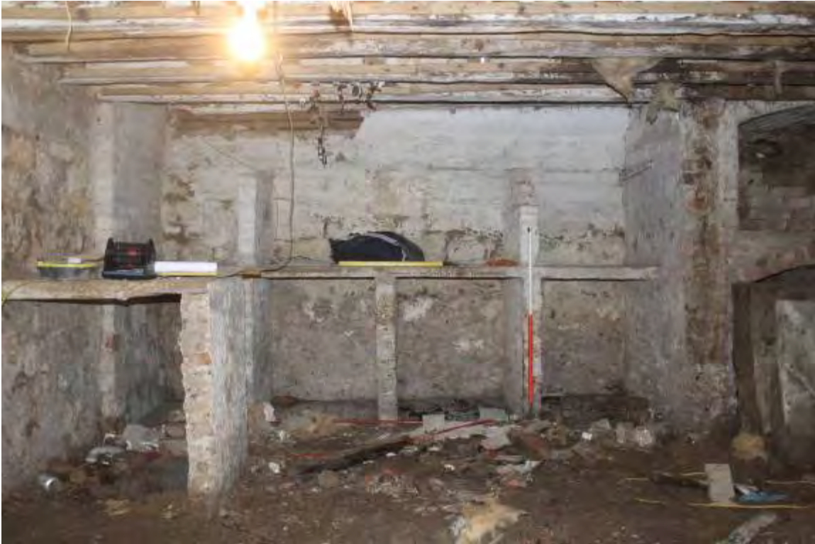
Brick and stone built wine bins against the E. wall of the cellar
