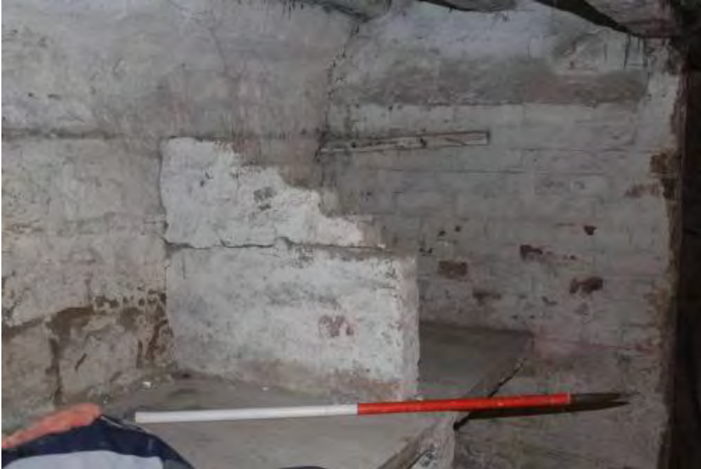
Photo 5. Timber batten against far wall supporting former shelf across top of brick dividers. Note "tide mark" on back wall at level of former upper shelf
