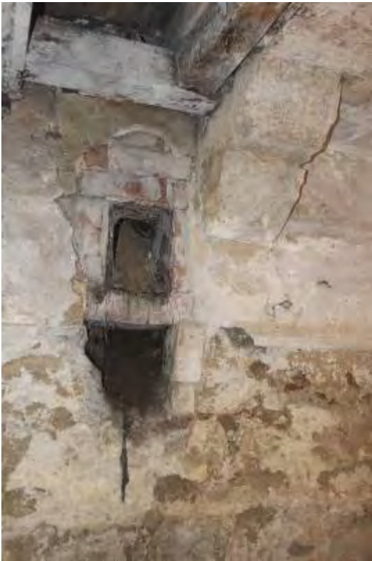
Photo 8. Vent and shute cut into cellar wall to LHS of fireplace above
