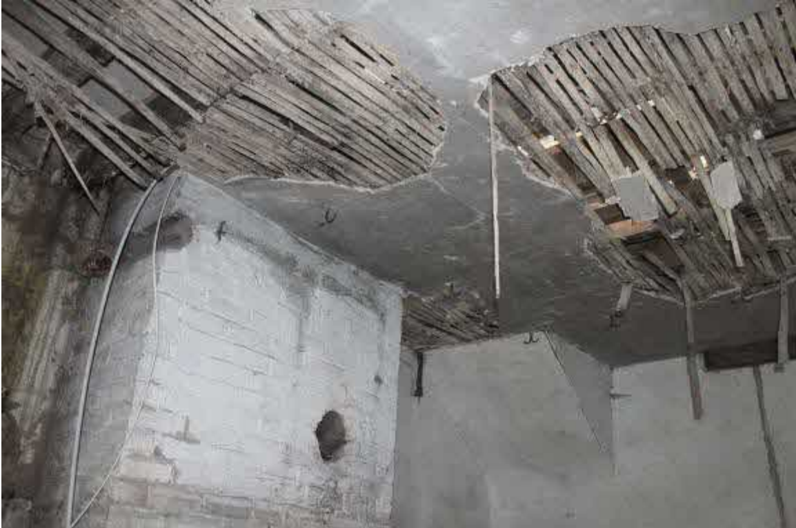
Large brick ?kitchen stack later used for coke/oil central heating boilers and hanging hooks in what remains of ceiling
