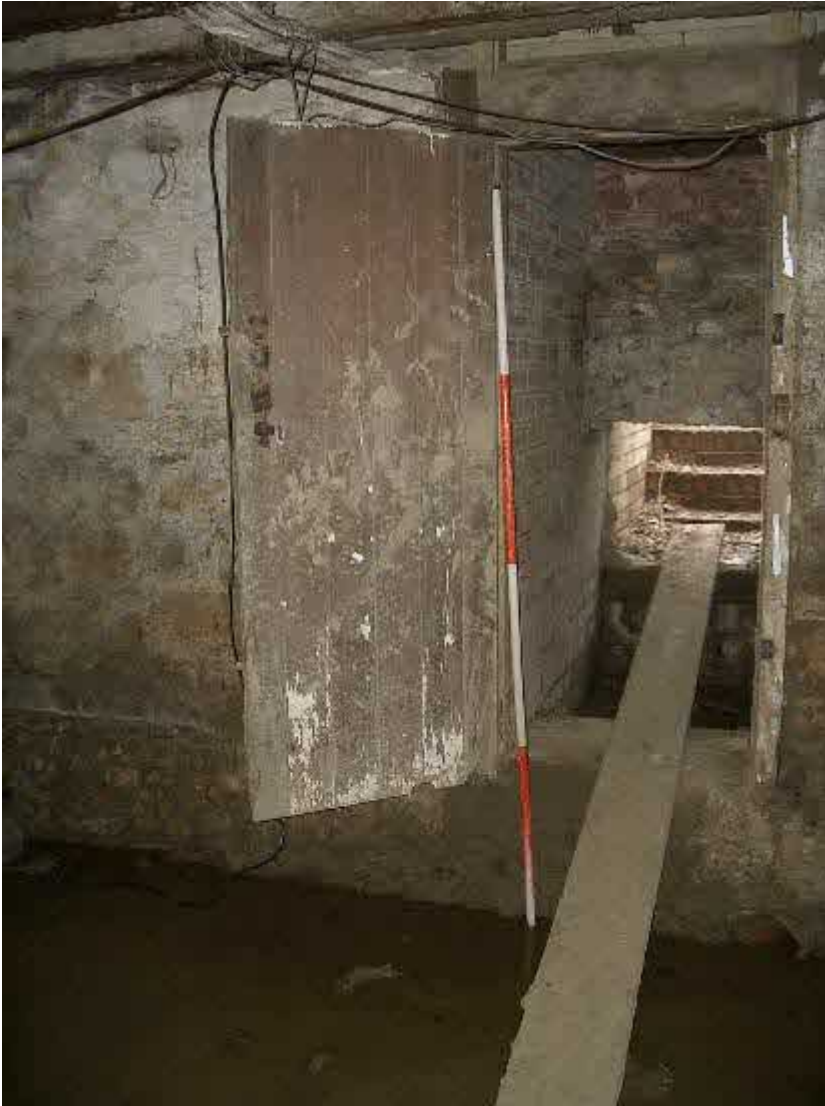
D53 leading S from 1880's cellar. Note height of threshold and excavation tidemark on walls, broken drain to R and "sump" beyond door. Steps up to garden terrace in passage beyond
