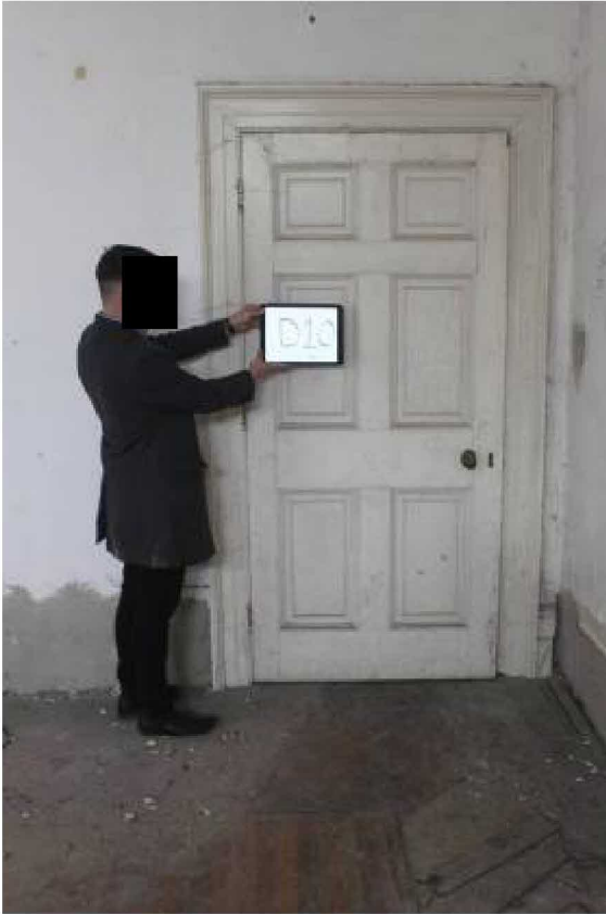
D10 inside Drawing Room. Some limited damage to parquet flooring (R)
