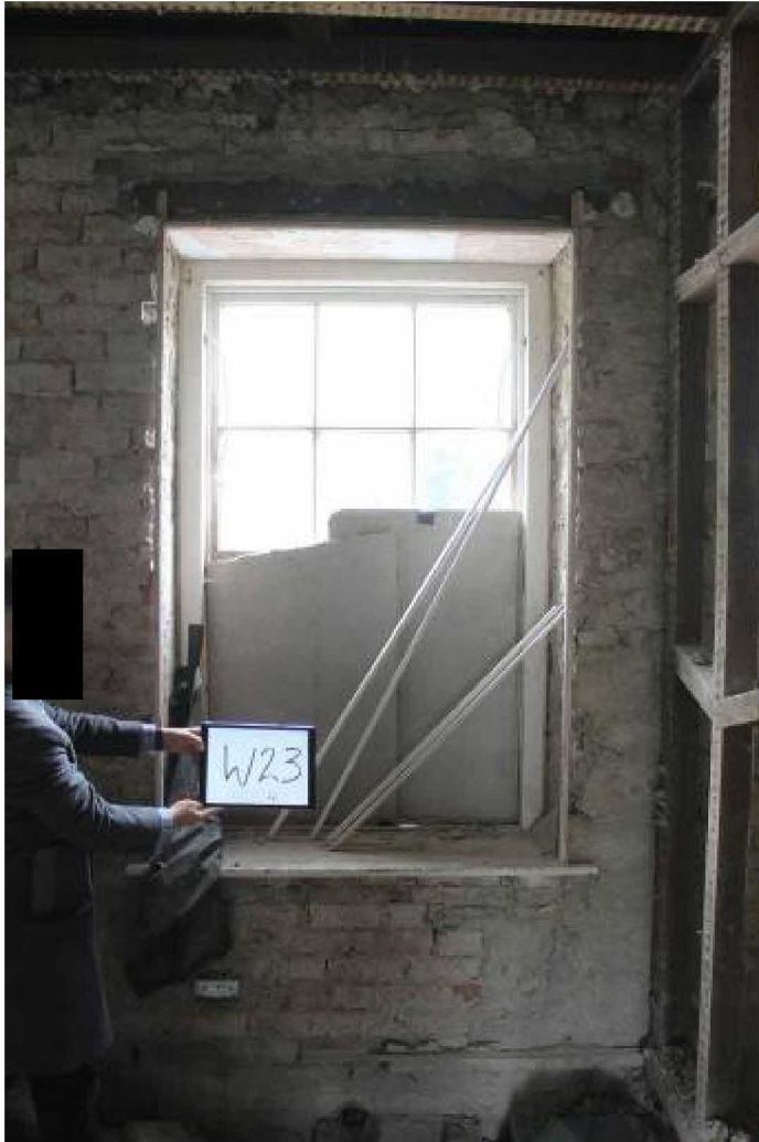
Much neater fit than W22, perhaps refitted into existing opening in 1930's?
