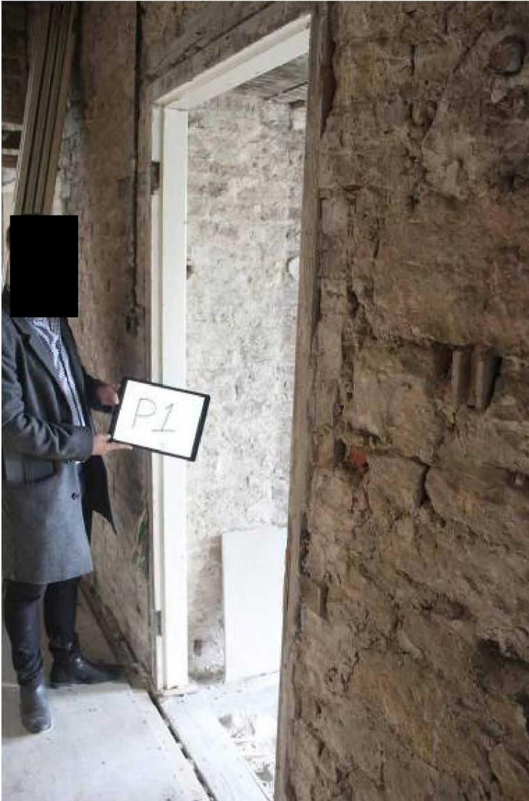
D28 off corridor To be blocked on room side to form cupboard (P1)
