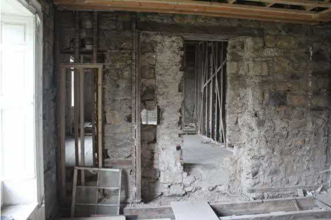
W wall. Timber lintel and brick infill of poss. window in rubble stone W elevation of Late C18/early C19 house. Modern breaches (to be infilled)
