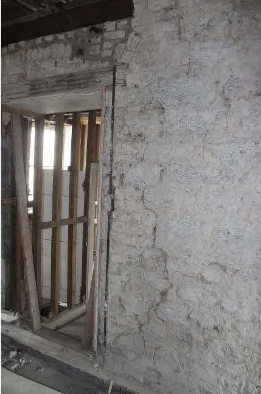
Ragged break in rubble stonework of late C18/early C19 build to R, Brick infill and relieving arch over change in level of corridor and beam above 1880's work
