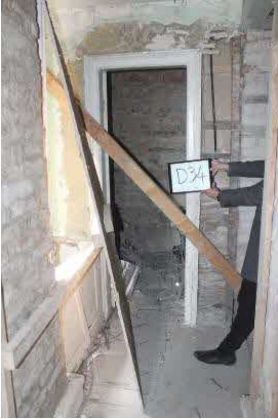
D34. Note cupboard below W26 to L.
