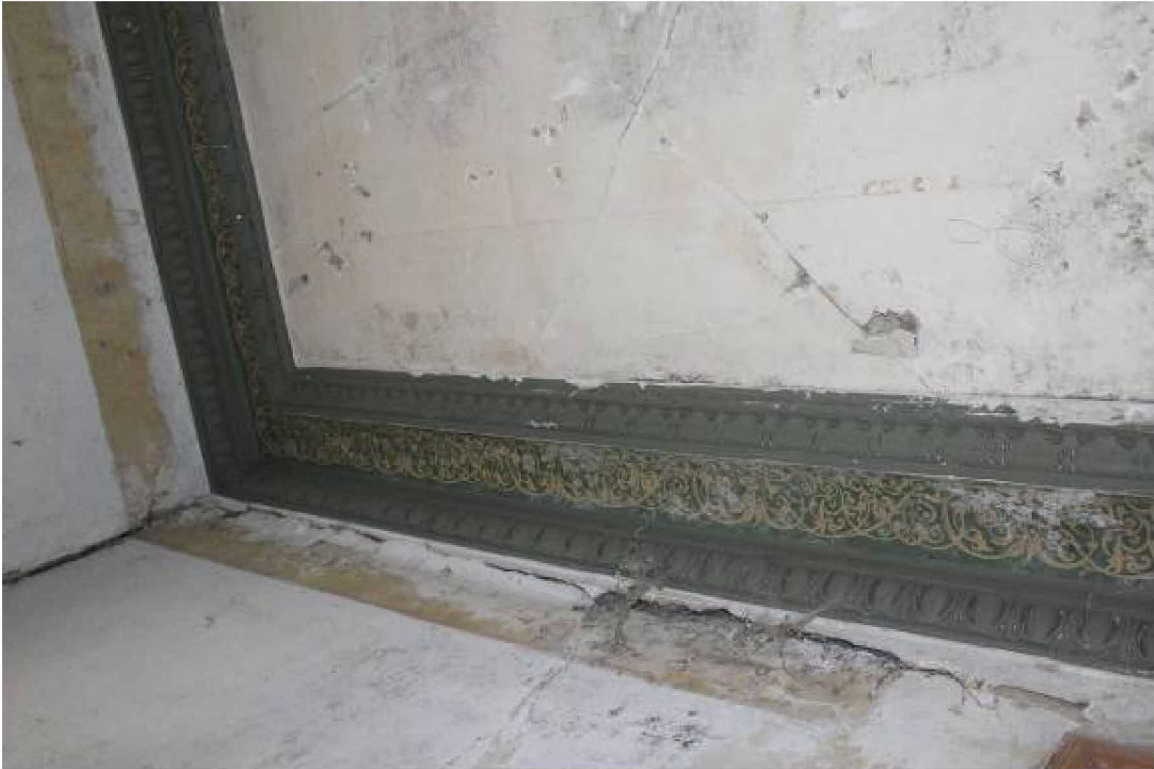
Cornice detail (badly damaged ceiling)
