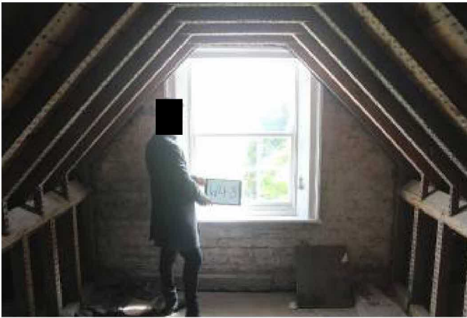
W48 in S facing 1880's gable. Note fixture R. Secondary glazing is proposed for the attic windows to improve insulation values
