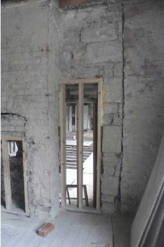
Breach cut through earlier S range stonework at angle. 1880s work to R.
