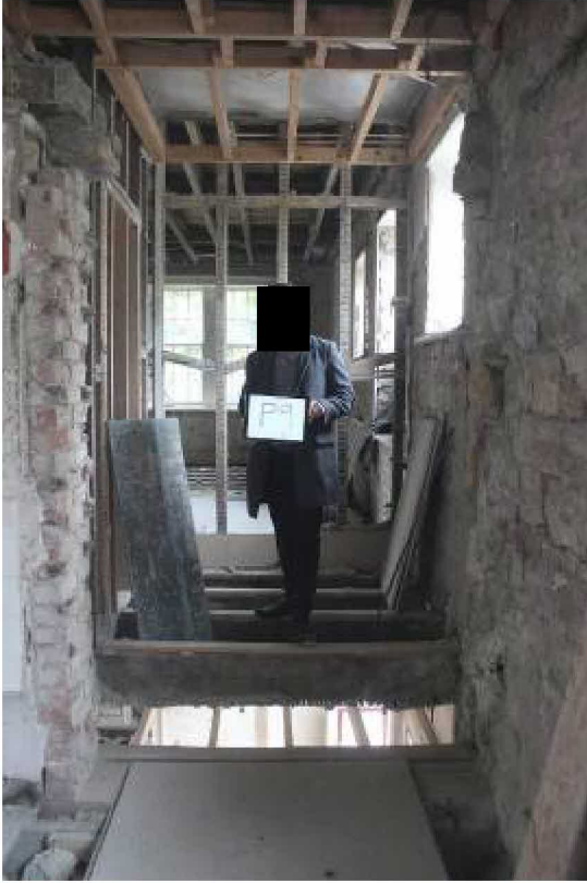
Location for new partition [P8] at W end bathroom. Note rubble stonework to R, brick to corridor wall L
