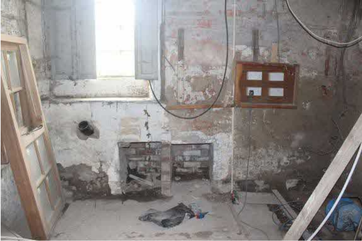
Blocked hatches in E wall may relate to late C20 use as dog room. DB's on this wall (house had its own electrical supply in 1880's).
