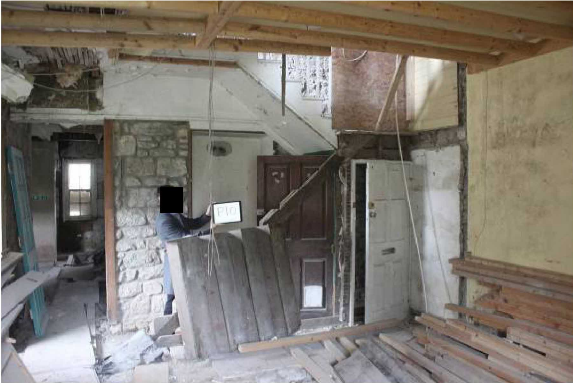
From former parlour looking NW towards remnants of lower flight of back stair and scar of landing, removed with partitions from stair and passage beyond in previous works. Note D17 (with letter box slot!) to right. Proposal 10 to reinstate stair and landing.
