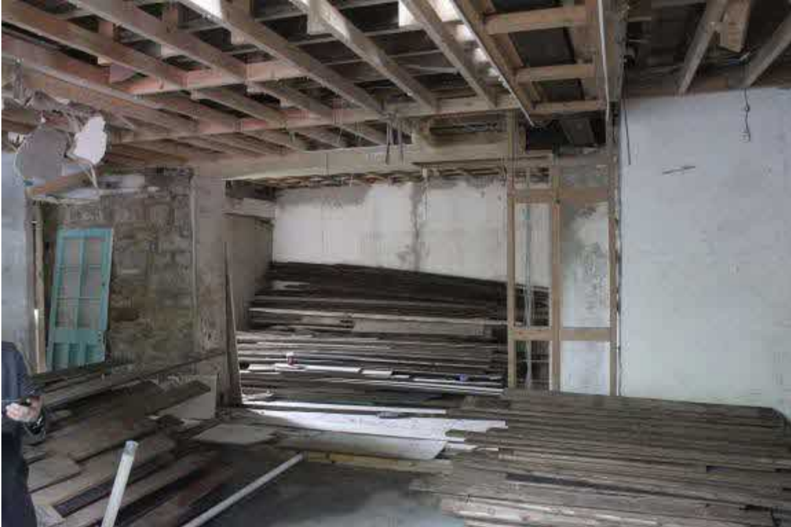
Modern opening in S wall. RSJs spanning (and also from RHS of opening to above viewpoint) when recent (2000's) kitchen made. Beyond the remaining wall (right) was a pantry, lit by W4
