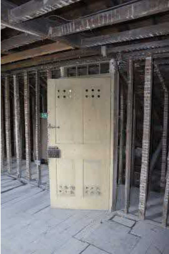
D45 room side with metal lock box. Note stubs of former internal partition on beam above
