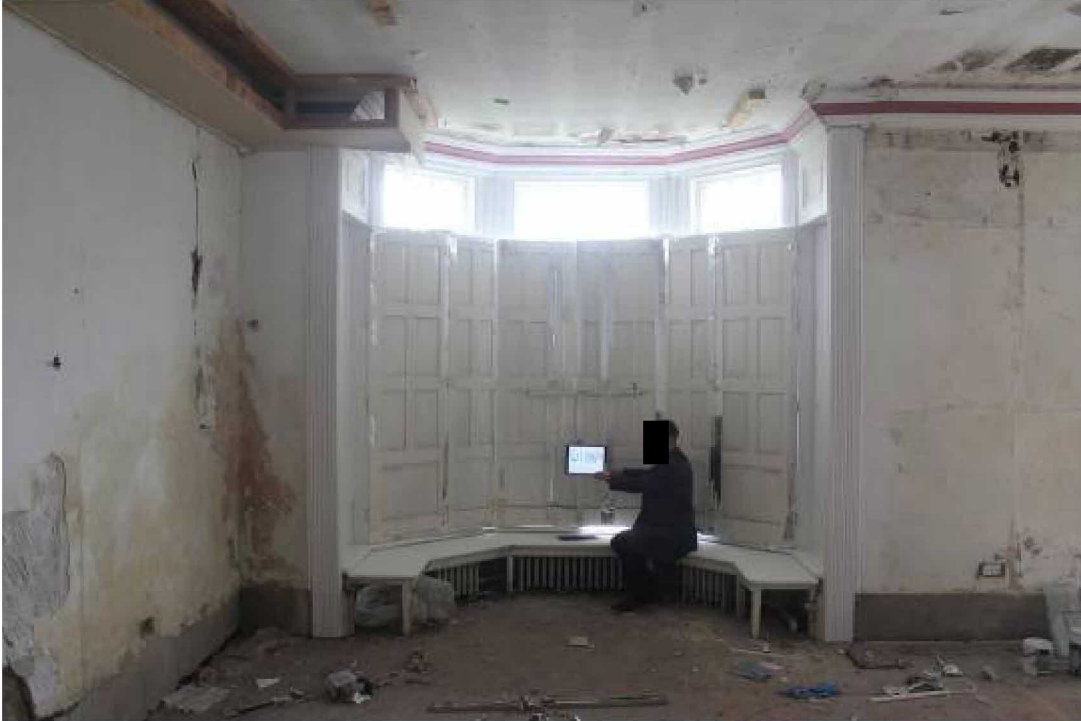
Shutters deployed within bay window. Note boxing in of cornice (top left)
