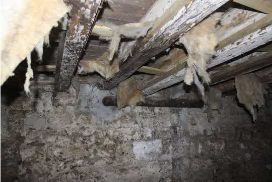
Roughly trimmed floor joists running to S wall of 1840's build. Iron pipe (?support for dropped joists) set into S wall
