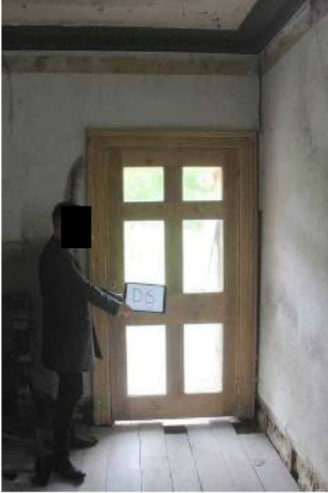
D6 Panels removed and glazed for modern access to late 1980's conservatory. Proposal GF4
