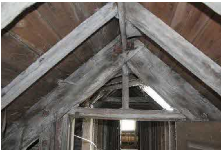
N attic roof. Bolted (?re-used/strengthened) truss with construction mark, III, on RHS looking S.
