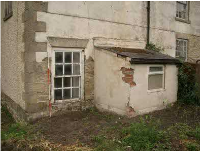
SE corner. Regular stone quoins. W10 C18 original (pegged sash/heavy glazing bars/no horns). 1960's scullery to be removed
