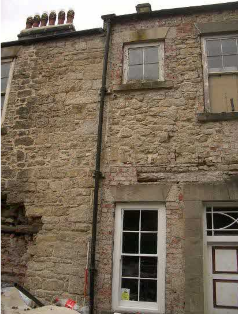
Build break to East of main door. Very irregular quoins. W2 & W24 above, inserted 1930's with doorway. Note blocked joist holes above embedded timber above door
