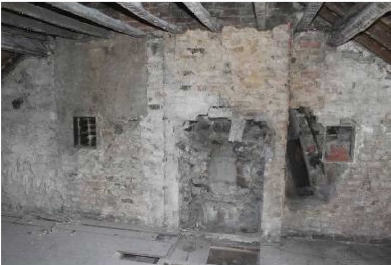
E gable of attic showing ceramic flues, leading up from FPs below, to R of FP12, and soot doors giving access for cleaning flues
