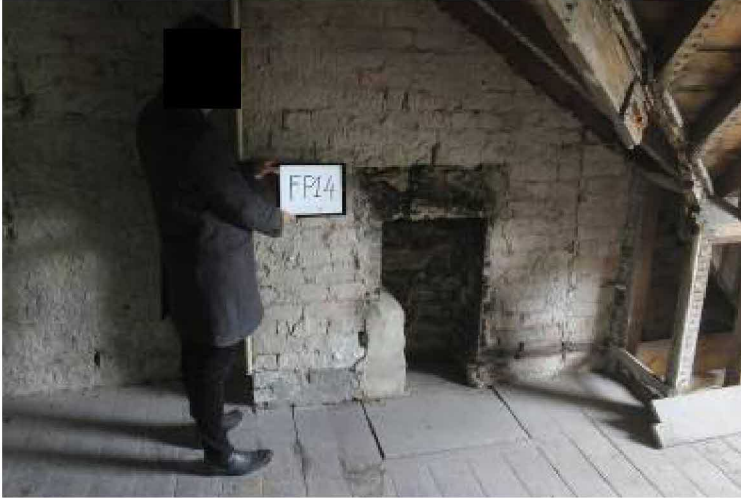
FP14 Modest 1880's attic bedroom FP. Note rot damage to roof timber to R.
