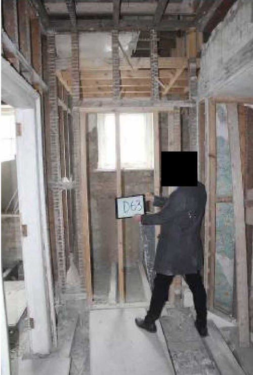
Proposed D63. W24 beyond. Surround for D23 to L Small area of ?C19 wallpaper to R
