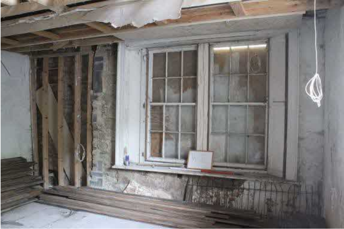
Large double sash window in W wall providing good light for billiards table in the large open space. Shutters LHS missing. 1930's alterations?
