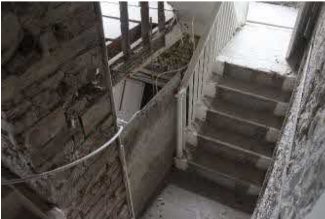
Passage landing and back stairs up to S. Proposal 14 to reinstate lower flight (void beyond board)
