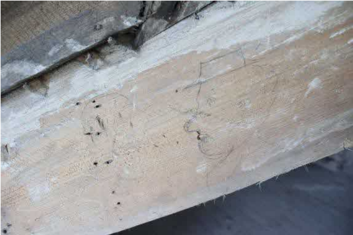
Graffiti on roof timber RHS W48
