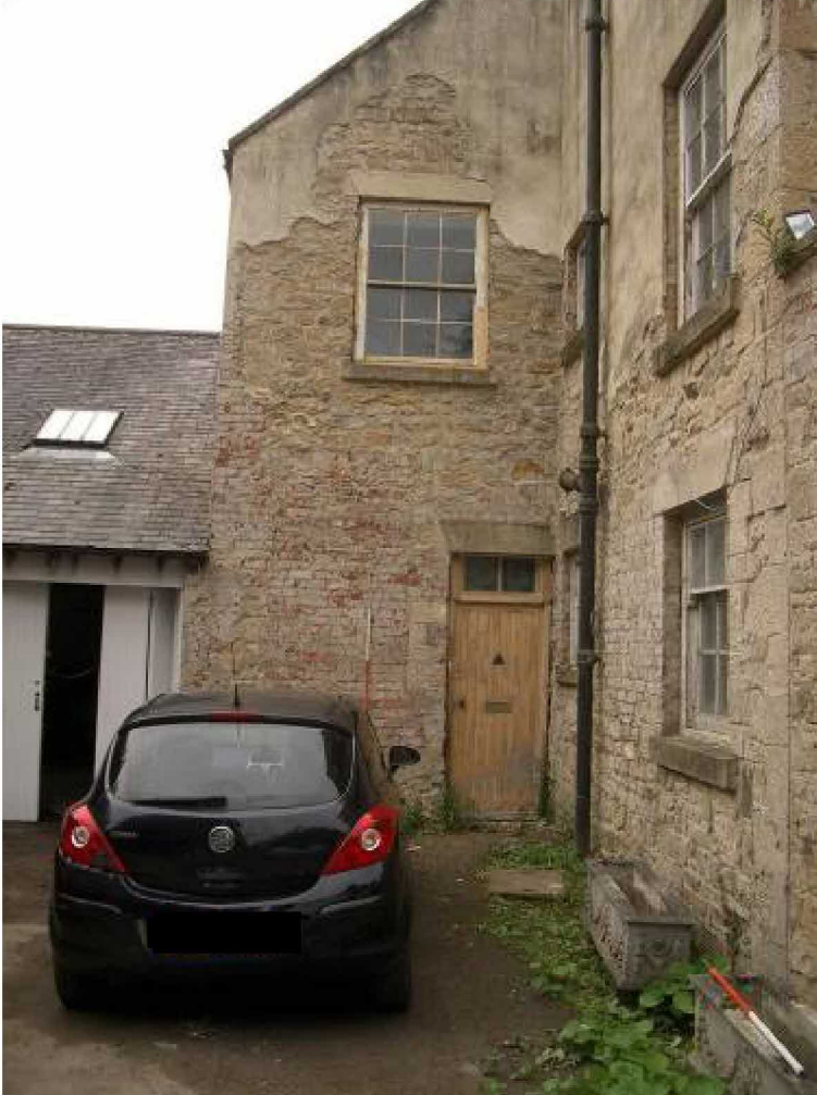
W end of C18 double span block in rubble stone. Note no quoins and ragged brickwork up LH return and poss. brick blocked opening behind car. W31 No horns on sash
