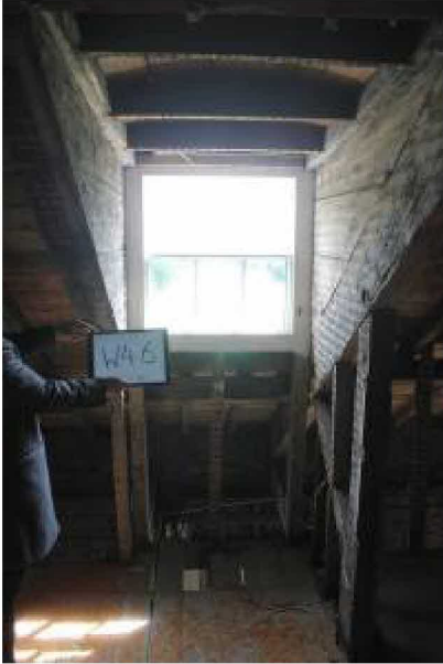
W46 one of three S facing dormer windows. Secondary glazing proposed for the attic windows to improve insulation values
