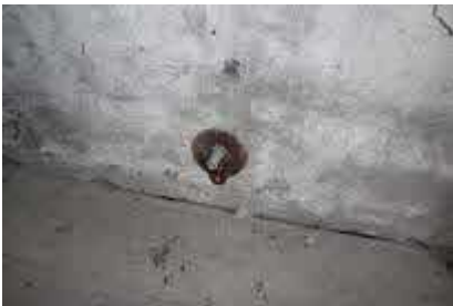
Fitting low down on N gable to RHS of chimney stack – tallies with external fitting - for wiring?
