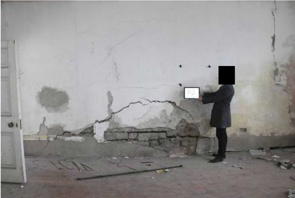
Settlement cracking in E wall due to breach made in cellar below Proposal GF2
