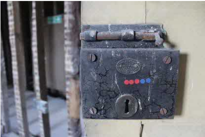
Lock on D45 supplied by Emley and Sons, Newcastle, a large late C19 supplier of house interior fixtures (may have included the now missing 1880's fireplaces).
