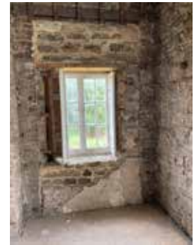
Photograph showing scarring surrounding window W36
