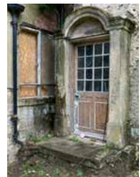
Photograph showing clash of window W11 with stone door surround
