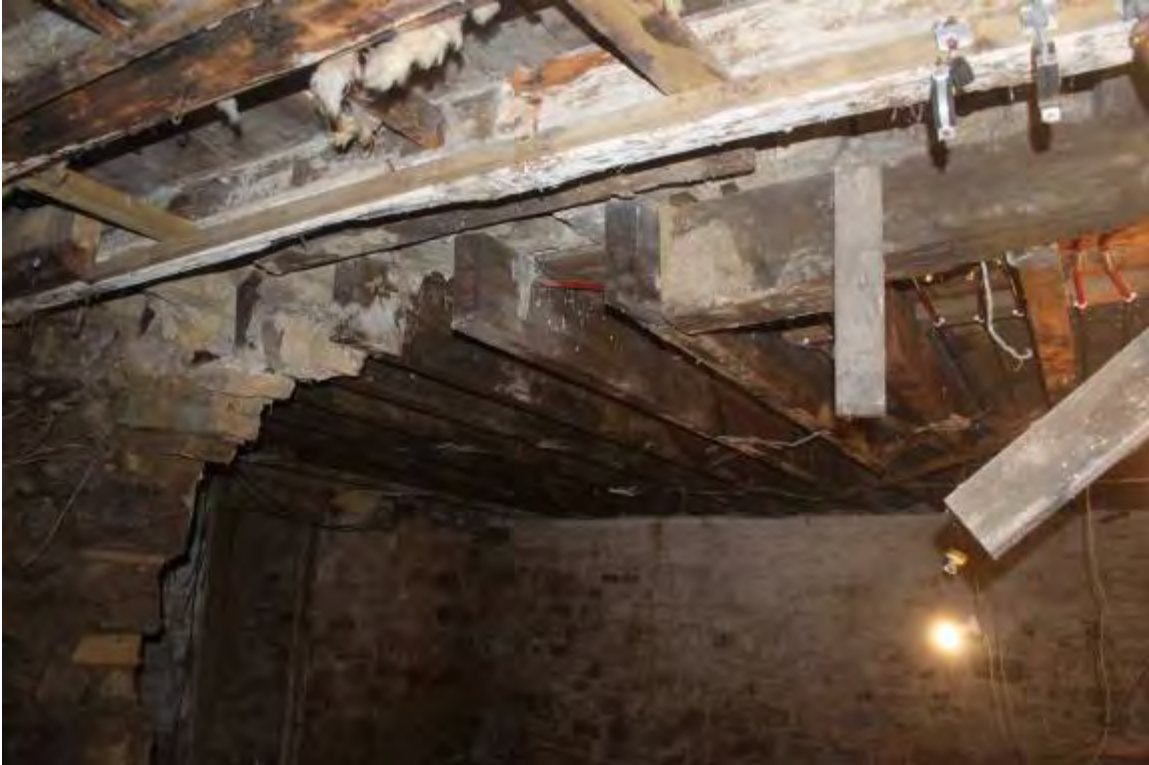
Photo 17. E/W running floor joists above 1880's cellar, left unsupported by removal of supporting cross wall
