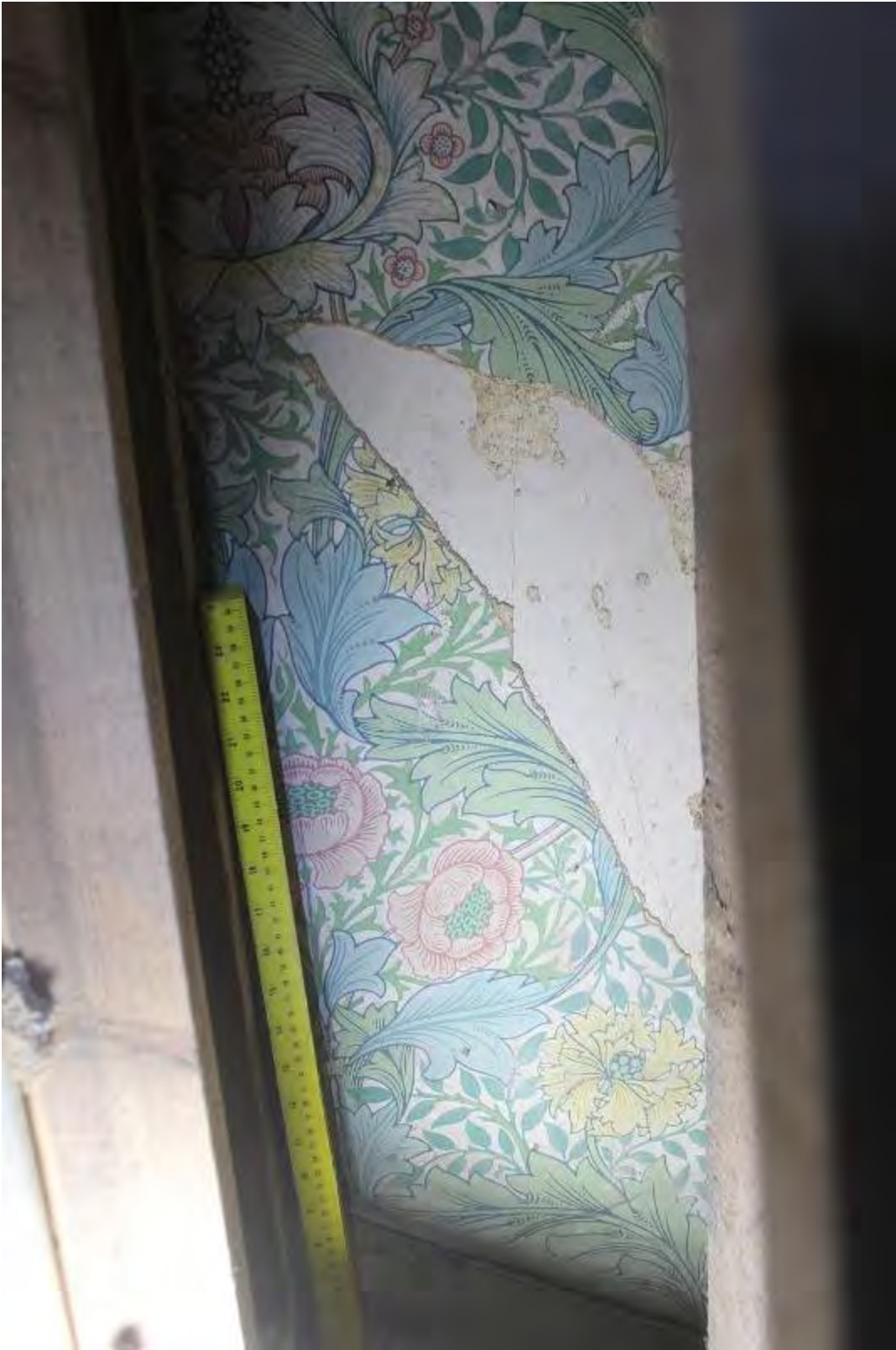
Photo 20. Lower section of wallpaper
