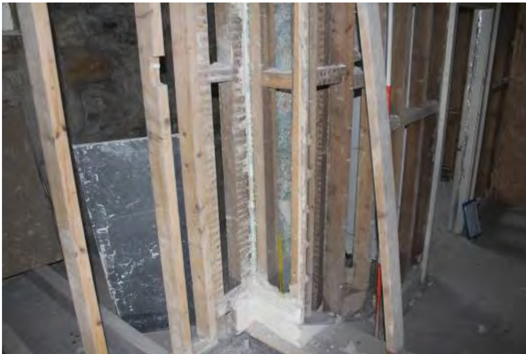
Photo 18. General context of wallpaper survival behind later studwork and plasterboard, looking NE.
