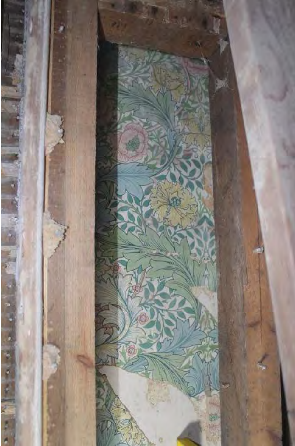
Photo 21. Upper section of wallpaper. Note remains of 1930's plasterboard adhering to later studwork overlying the wallpapered wall. Earlier studwork partitions (left of view) are traditional lath and plaster
