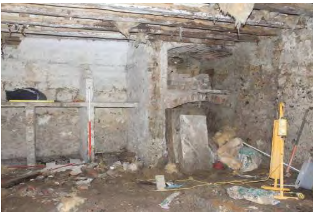
Photo 4. Arched wine bins built in brick against southern wall. Note floor joists running N/S across cellar
