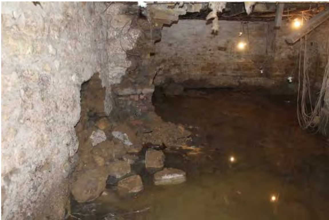
Photo 12. Stub of cross wall removed in previous works and recent collapse of unsupported south wall. 1880's cellar in background
