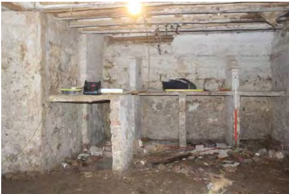
Photo 3. Brick and stone wine bins built against east wall of cellar. Stone shelf in front of bins left middleground
