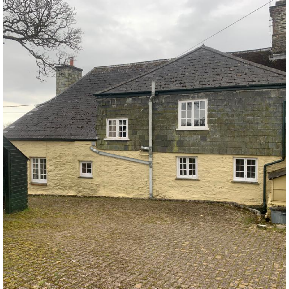
10. Rear Elevation Proposed - New soil pipe existing near current BT connection and joining the existing soil pipe
