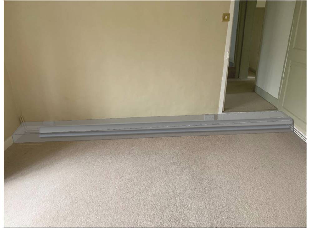
04. Bedroom 2 Proposed - Pipework to run at floor level and boxed in. Existing step to be extended.
