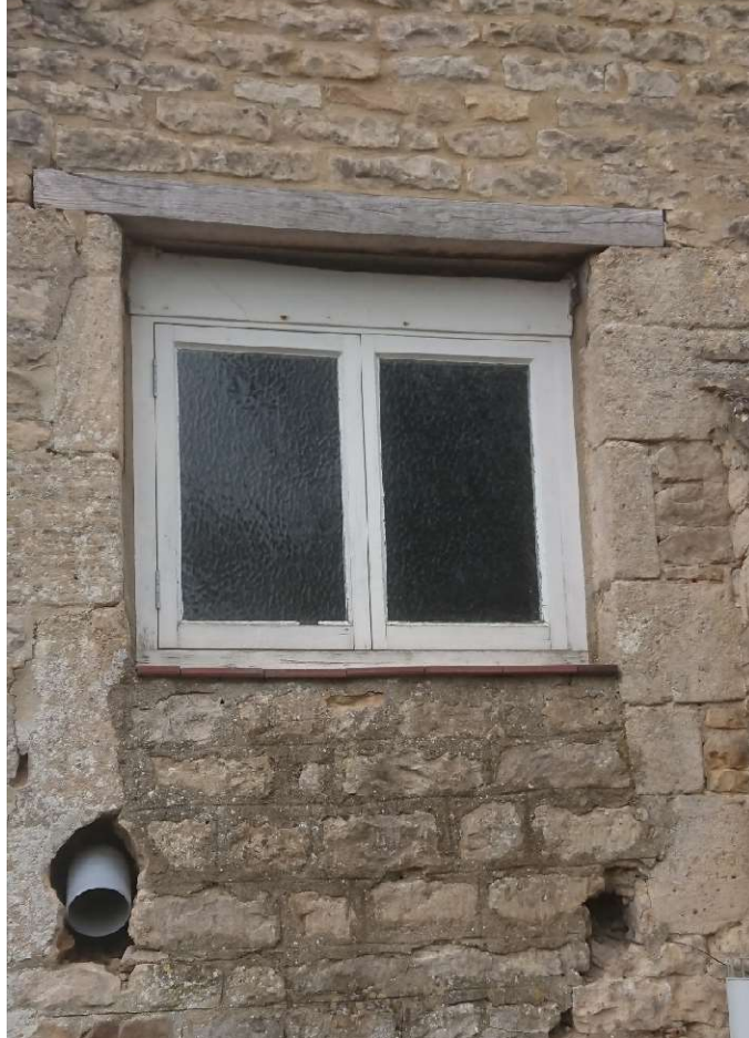
Photo 11: Bathroom Window and In-fill Below
