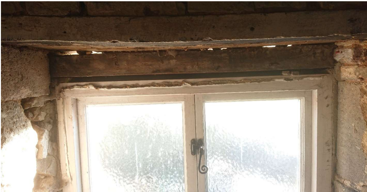
Photo 12: Old Doorframe Head in Bathroom Window Opening (showing poor window fitting)
