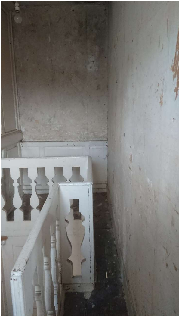
Photo 10b: Wasted Space and Narrow Access
