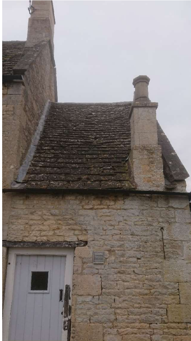
Photo 7: Lower Range Roof (showing damage)
