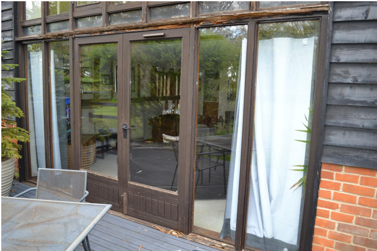
Plate 3 - Note the damaged threshold and significant degradation at the head of the doors and sidelights.
