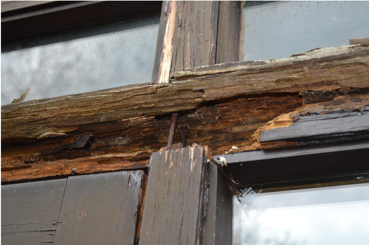
Plate 4 - Extensive Damage - Replacement with hardwood joinery will offer superior lifespan.
