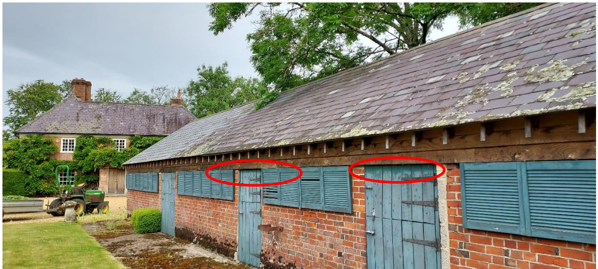
Photo 12: Gaps at the stable doors
