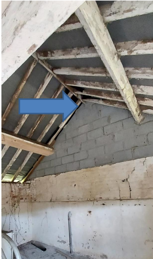
Photo 4: Gaps for bats between different internal rooms
