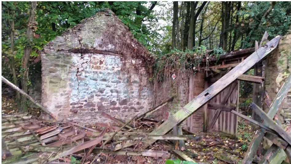
Figure 12: After the night of the collapse, the barn's one remaining complete wall.
