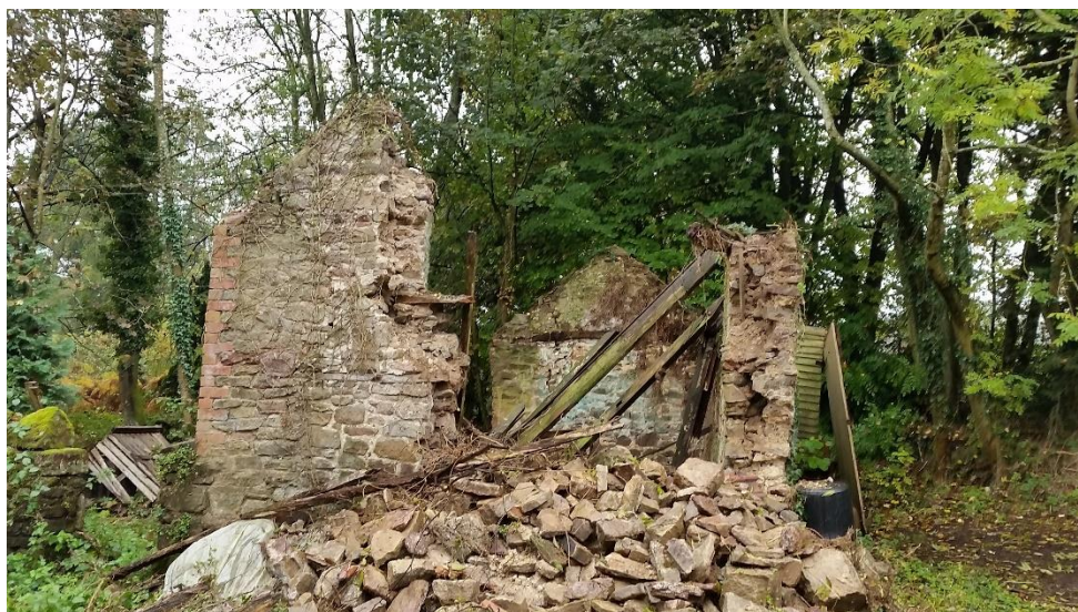
Figure 13: After the night of the collapse, this wall had been intact the day before this photo
