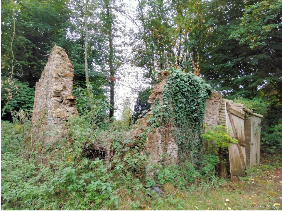
Figure 9: The remains of the original barn after its roof structure and some of its walls collapsed in 2020.
