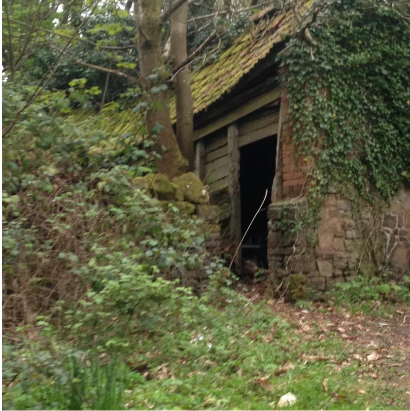
Figure 7: The Folly barn in 2018, with the sycamore tree growing in front which ultimately undermined the whole building.
