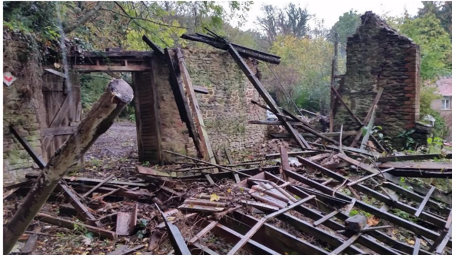
Figure 11: After the night of the collapse, the roof structure lies across the ground.
