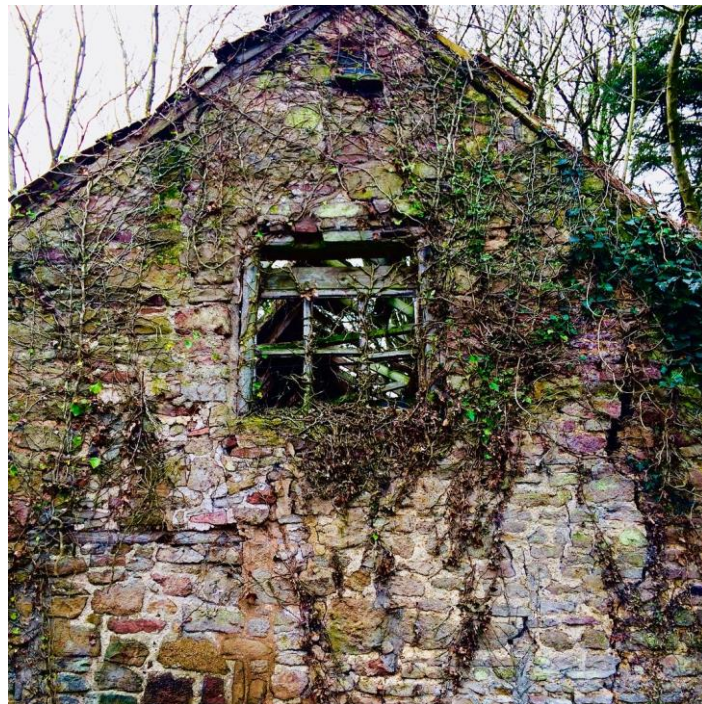
Figure 8: Original stonework & roof tiles of the Folly barn, before its partial collapse.
