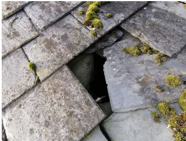
Photograph 5: Slipped tile and ripped felt lining below provides a large access hole into the storage room
