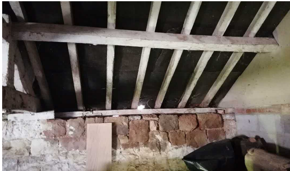
Photograph 11: Gap in felt lining above the wall plate on the eastern boundary
