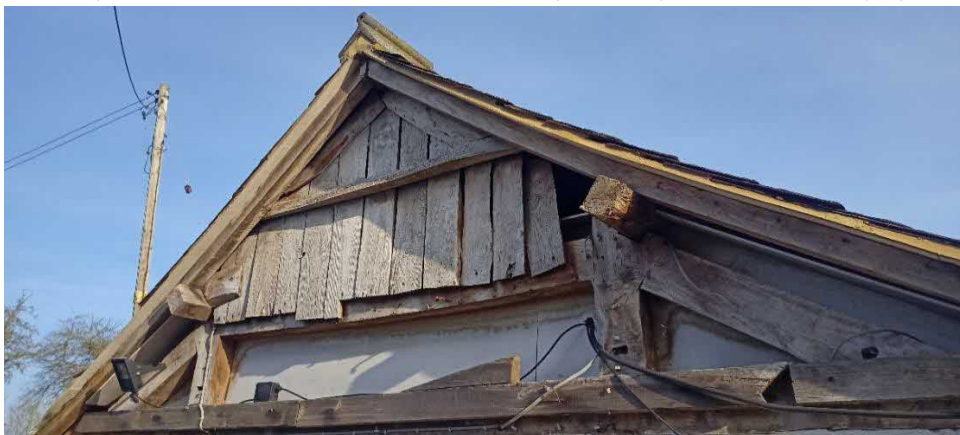
Photograph 3: Western end of the outbuilding where hip has previously been demolished. Gaps present between the wooden slats allow access into the roof void above the boiler room
