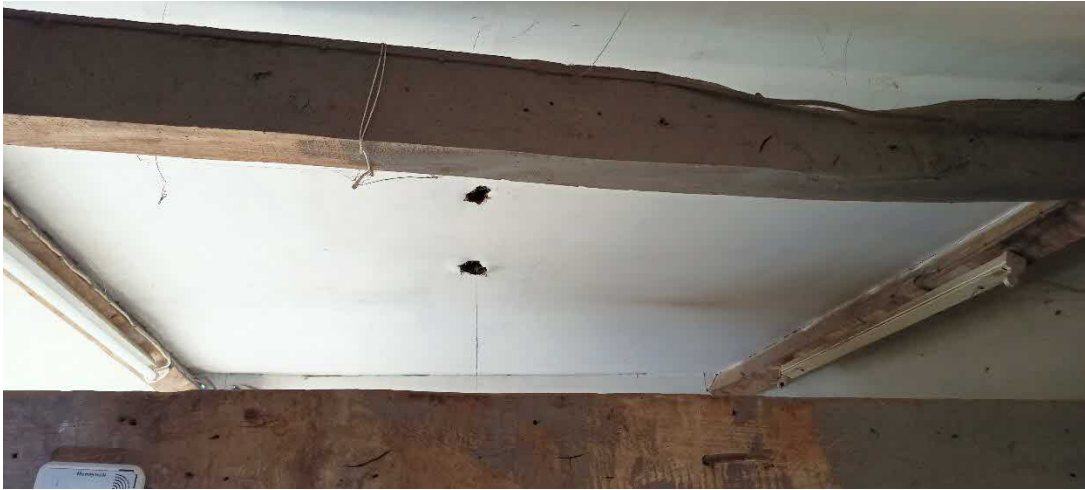
Photograph 7: Holes within the ceiling board within the boiler room
