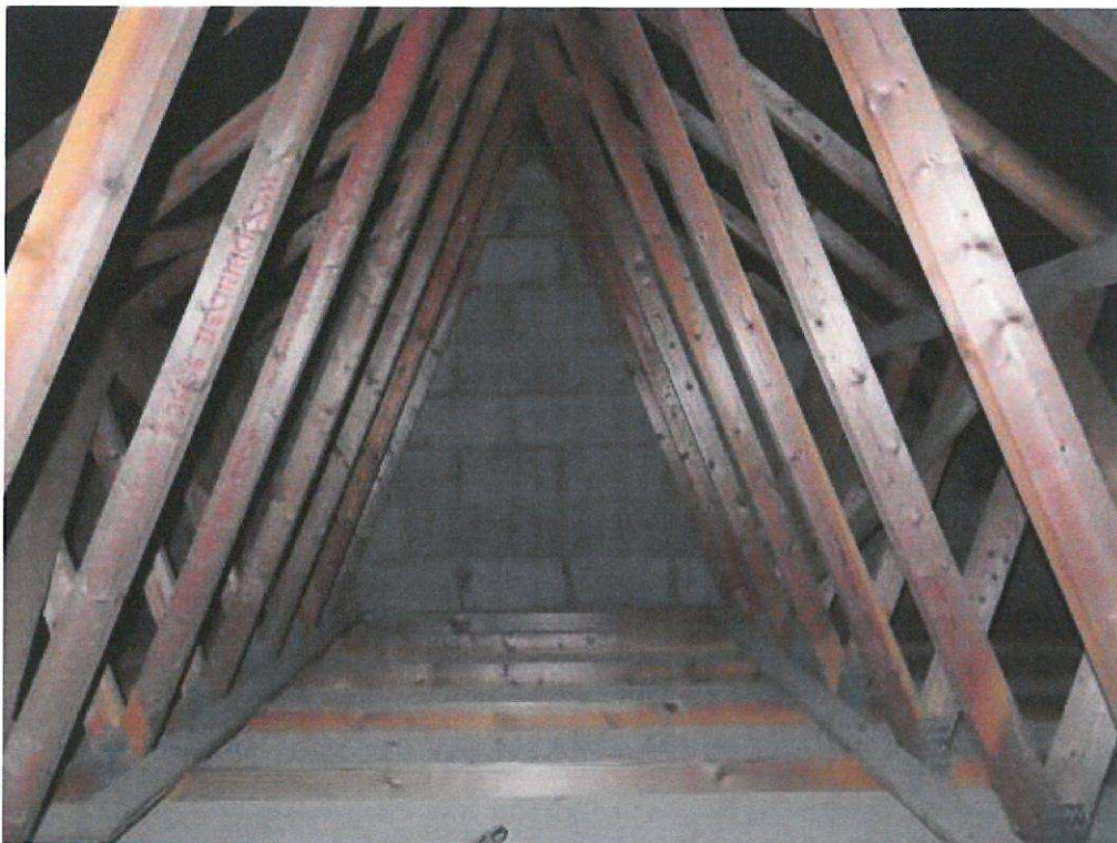
Photograph 6. Interior. View of party of the roof-space above the car-port. Looking northwest from southeast.
