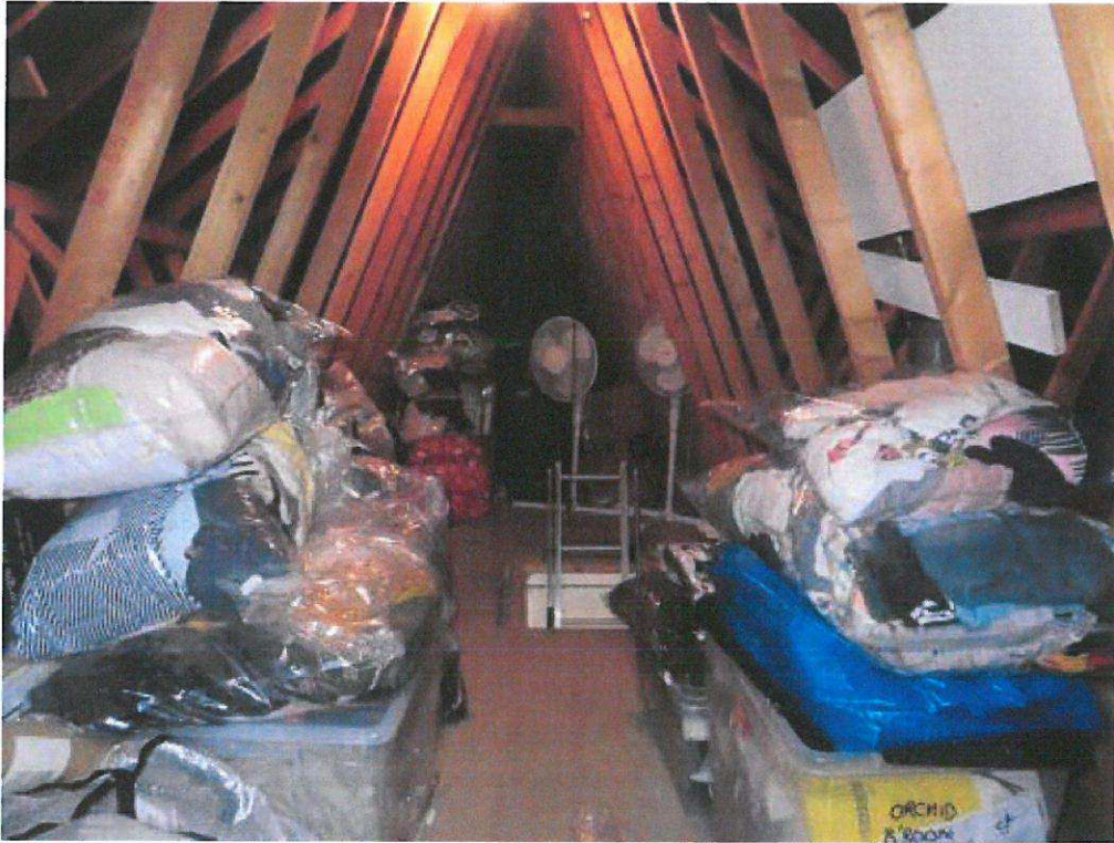
Photograph 5. Interior. View of part of the roof-space of the main, two-storey, section. Looking southwest from northeast.
