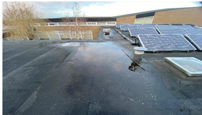
Close-up on Roof1a of ponding water surrounding the existing penetrations and plant.
