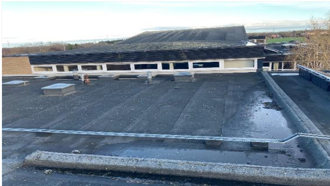
Overview of part of Roof1a – as shown areas of ponding water and moss/vegetation are evident.
