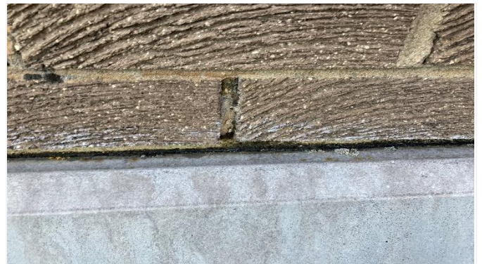
Existing Lead flashing is splitting away from the brickwork causing exposure to the building
