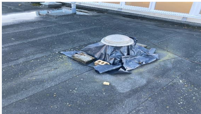
Existing penetration has been exposed and temporary coverings have been placed over and require immediate attention
