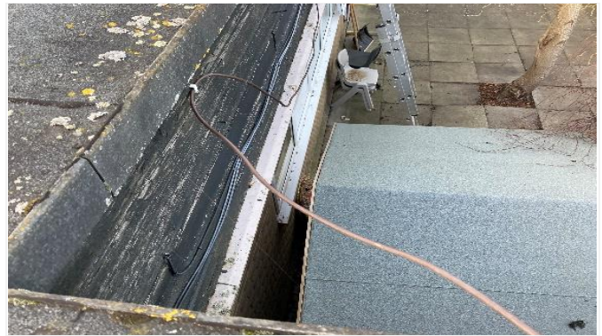
Check kerb detail shows signs of cracking and exposure. Poor condition of fascias also evident here
