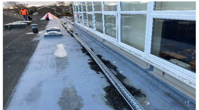
Part of Roof1b shows repair work evident along with ponding water and moss/vegetation
