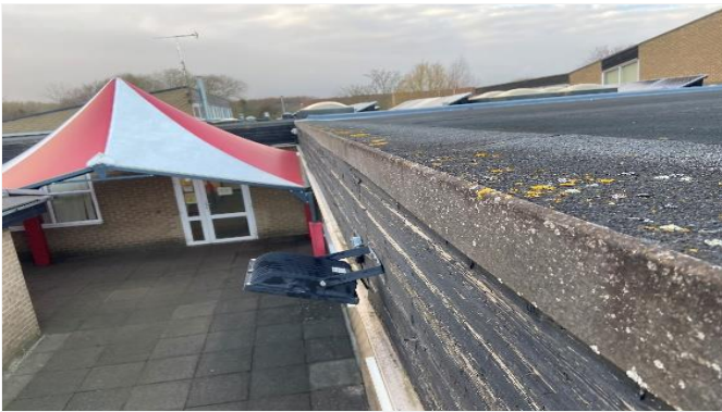
Existing fascias are also in poor condition and will require work
