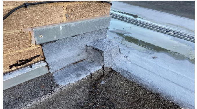
Repairs on Roof 1b upstand detail are evident and not sufficient
