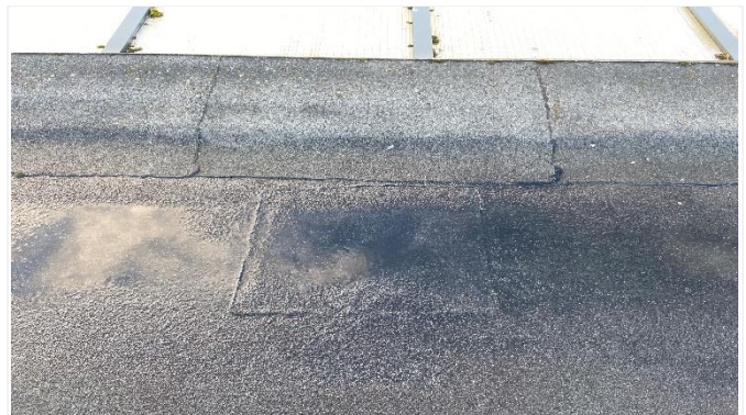
Some outlets have been discarded, this has created ponding water in areas. These details need reinstated.
