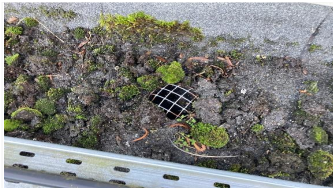
Existing outlets are blocked due to moss/vegetation
