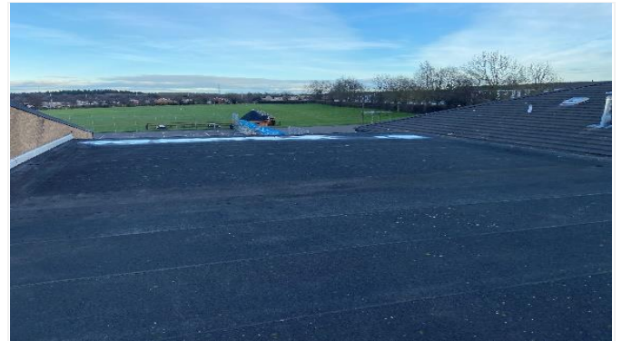
A second overview of Roof1a – Ponding water evident
