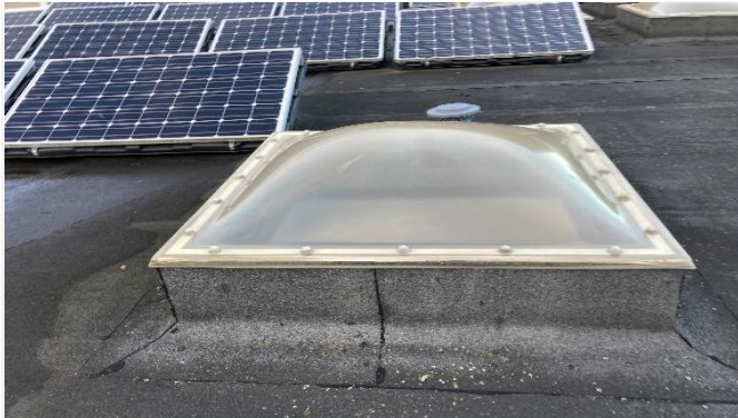
Existing rooflights are not in accordance with current regulations and will require replacement.
