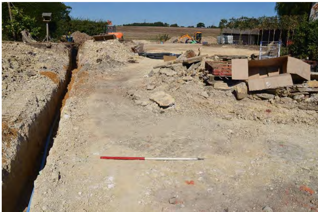
Plate 7: Feature [4] pre-excitation. Service trench visible on the left of photo. View west.
