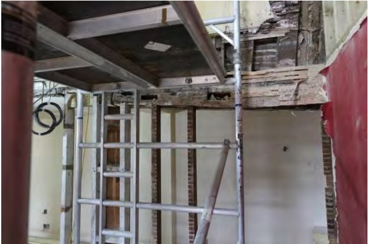
Plate 59 Extant mid rail and later softwood studs to lower register in new stairwell (F7A/F8)
