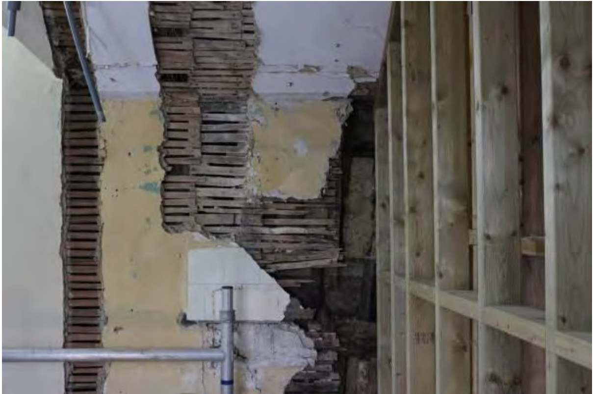
Plate 63 West wall of former ensuite (F7A), showing historic wall fabric behind lathes
