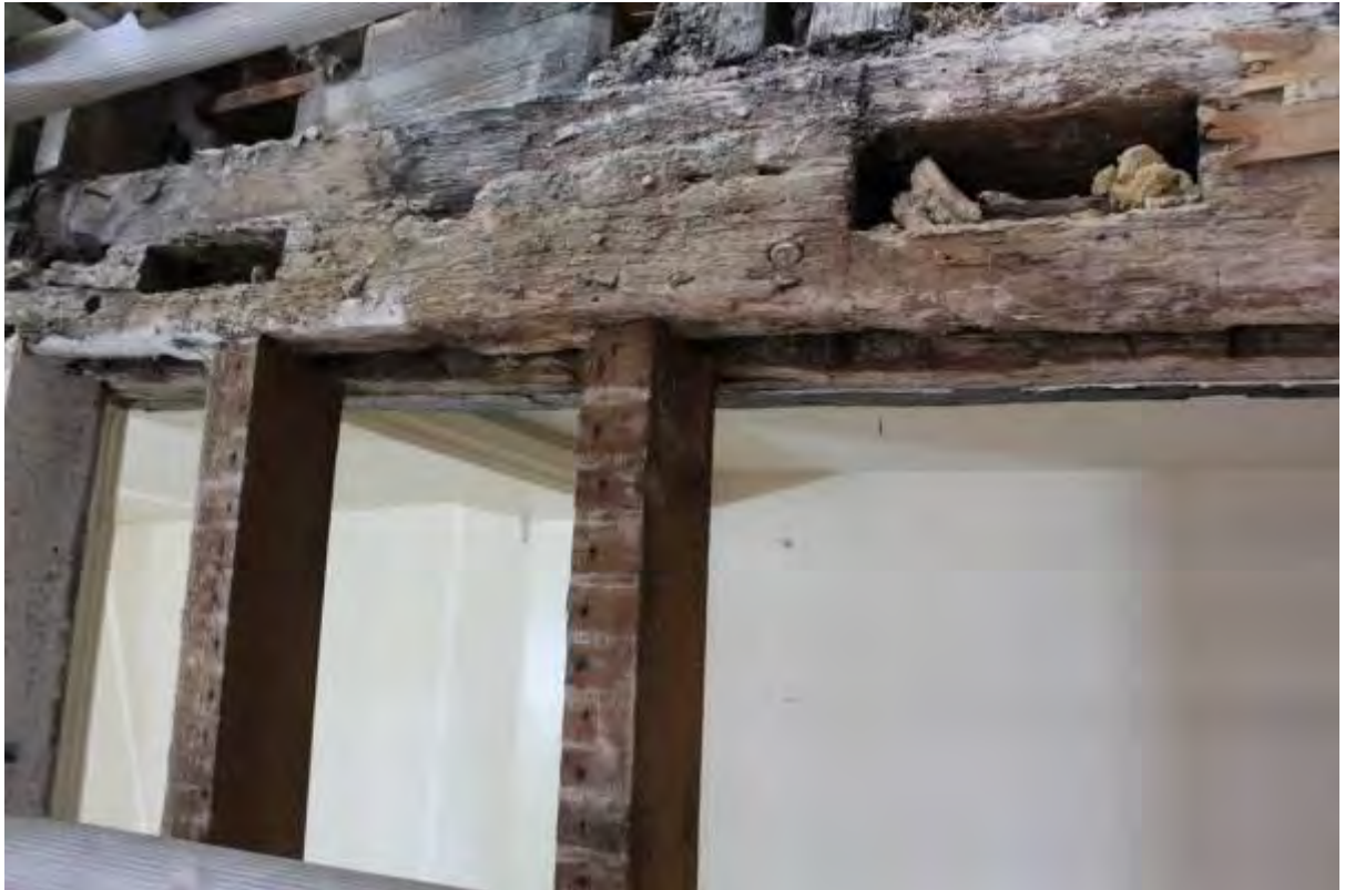
Plate 61 Two empty mortices associated with a later floor built as part of the stair tower
