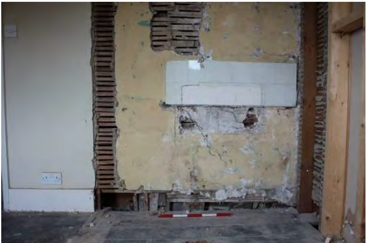
Plate 56 Base of historic wall studs seen along base of wall in (F7A).
