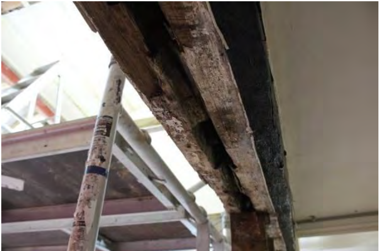
Plate 60 Empty stud mortices and trench for wattle panel cut into mid rail soffit
