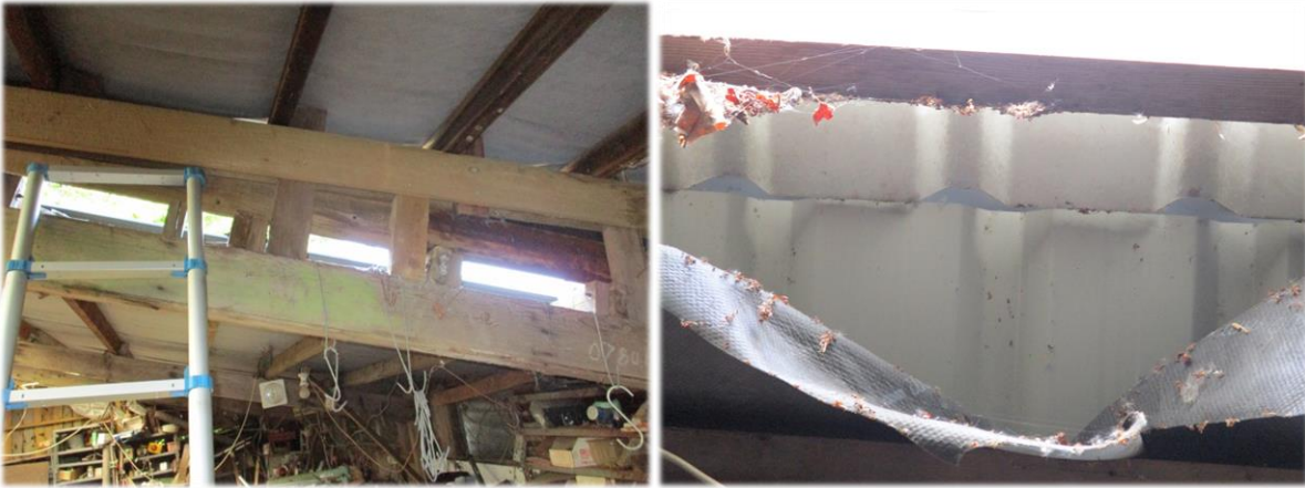
Storage barn gaps between adjoining roof sheets (left) and open ridge (right)
