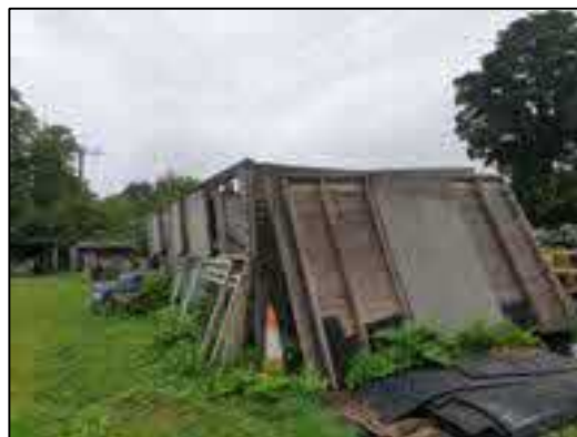
Figure 8 - Timber sheds, no roof
