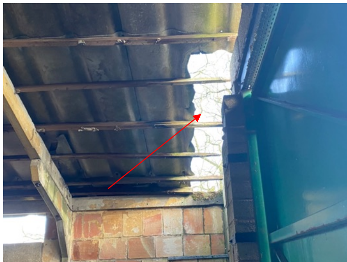
Photograph 11: Hole in the roof at the southeast end of the building.
