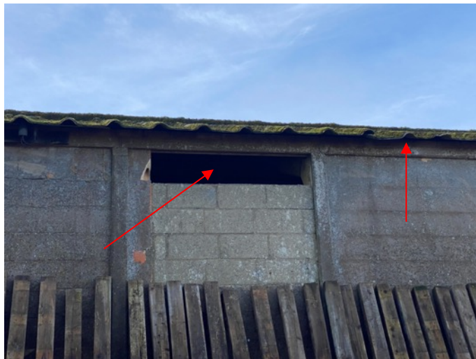
Photograph 10: Gaps under corrugated roof sheets and through wall openings.
