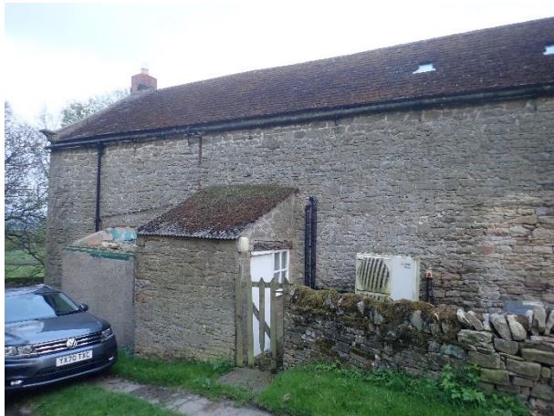
Kitchen area with no roof
