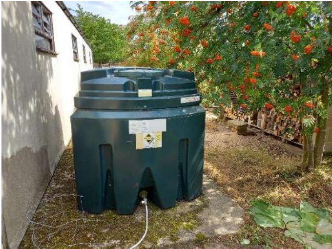
Figure 4: View of self-bunded oil tank.
