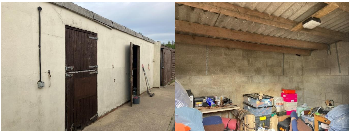
Fig 4 & 5. West elevation of stables B2 (left) and internal view of equine store (right)
