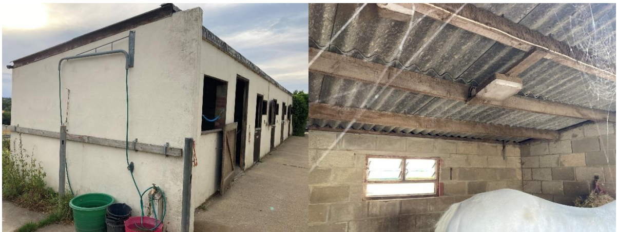
Fig 6 & 7. South and east elevations of stables B3 (left) and internal view of stable (right)
