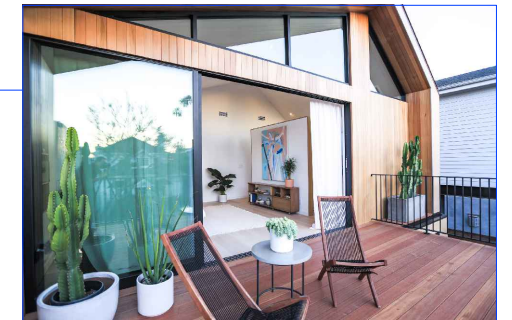
Roof Overhang and return south wall to project beyond main building line to provide privacy and protection for the balcony. Soffit and return to have continuous. Cladding to be board and batten style.
