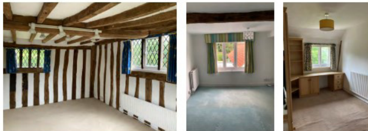
top views of exposed historic timber frame to Hallway and Sitting Room. The latter also showing the flatness and character of the C20th wall finishes middle left details of notable timber framing joint, centre/right views of framing to old farm office and to first floor corridor below views of framing to south bedroom with retained leaded-light windows, and other bedrooms with limited or no exposed framing
