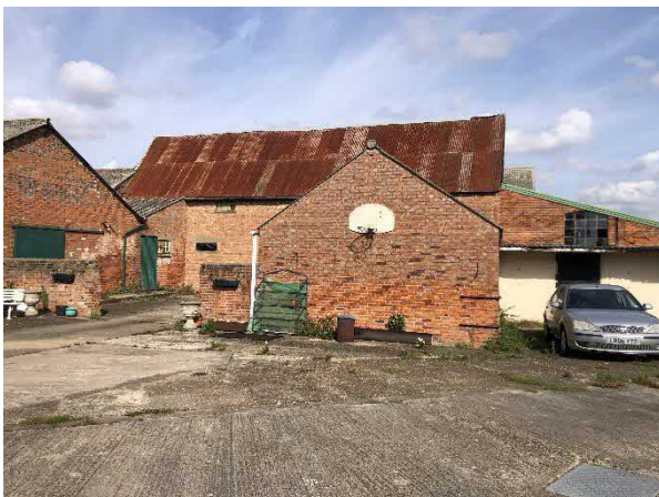
Photo 11: Southern gable end of B7, with tin roof of B6 immediately behind
