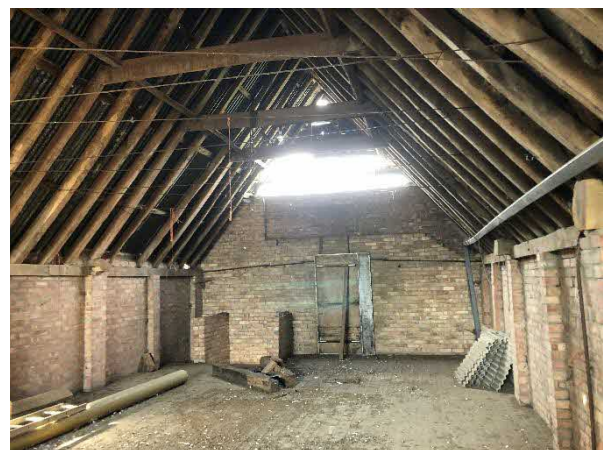
Photo 14: Internal view of B6, upper floor. Brickwork to eave height, and above eave height at the gable ends. Wooden wall plate rest: brick walls
