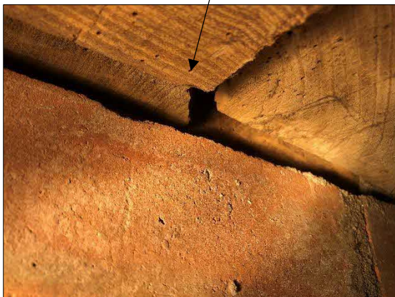
Above: location of confirmed common pipistrelle roosting crevice on the southern wall, in a gap between two adjoining wall plate beam sections (Sample 7 – S Wall), as indicated by red arrow
