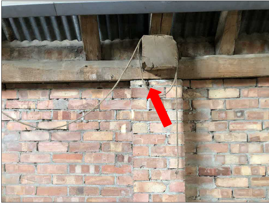
Left: location of confirmed features in north west corner of the barn (Sample 6 – NW Wall), where 8 common pipistrelle droppings were recorded beneath a clean crevice between the brick column and wooden wall plate
