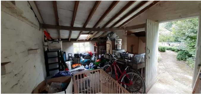
Roof of existing Garden Store that requires attention
