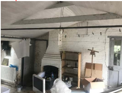
Existing chimney on west side of existing Garden store which will be retained and extended. (This picture shows the previous garage building which was removed as part of previously approved works)
