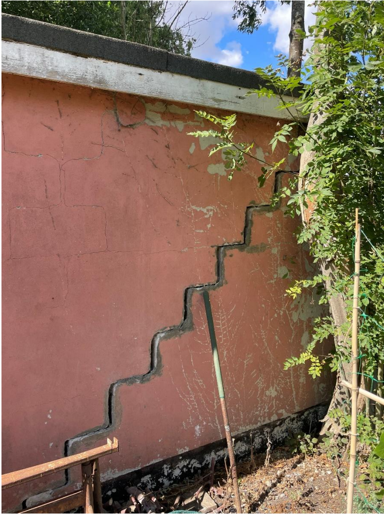
Image 2 – Cracking to garage
