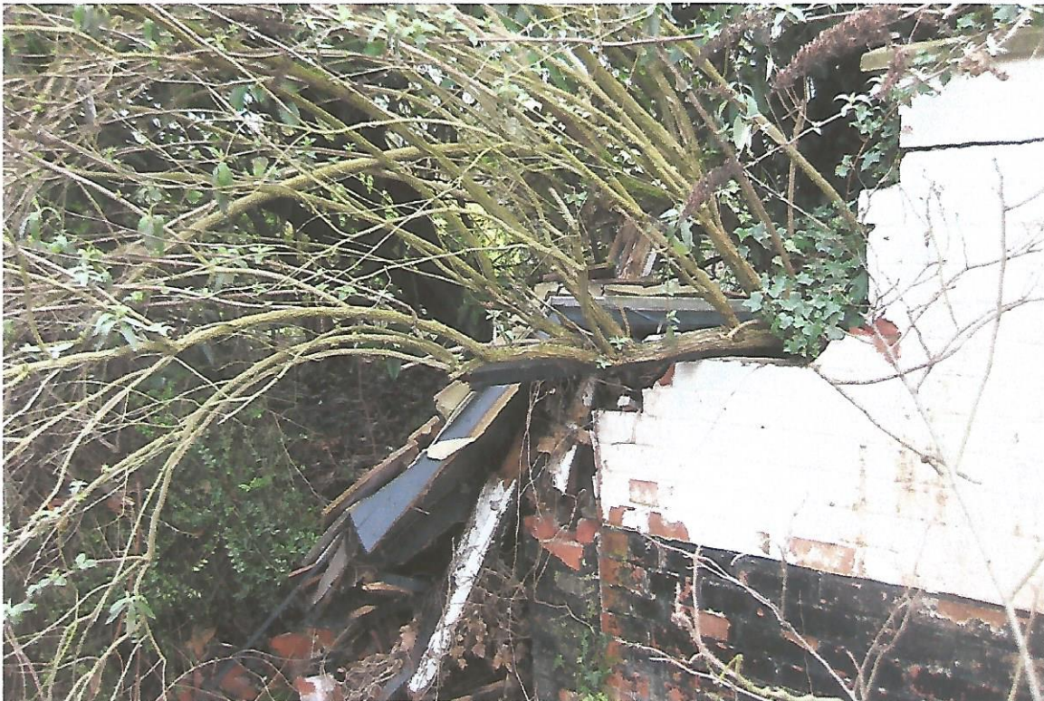
Picture 2 Damage to brickwall and lychgate looking from road
