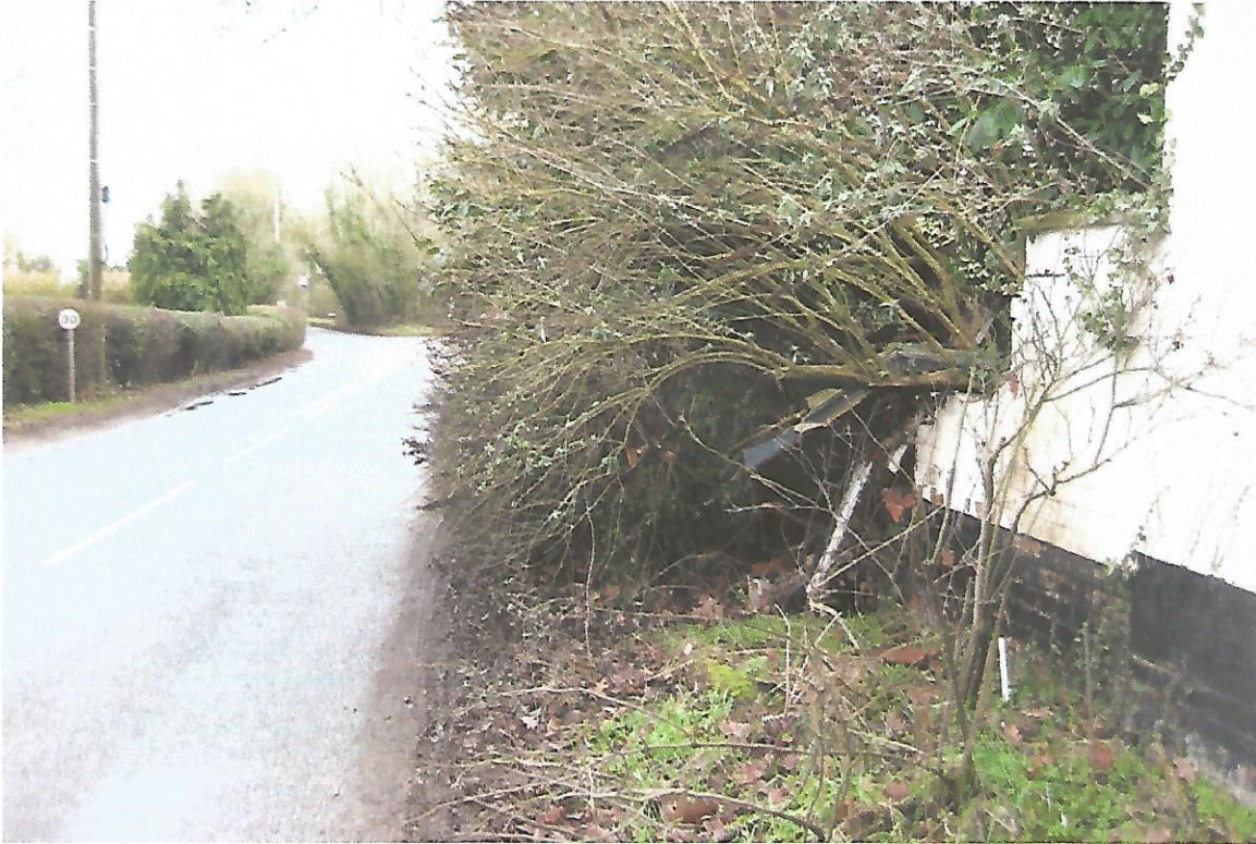
Picture 3 Damage to brickwall and lychgate looking from road
