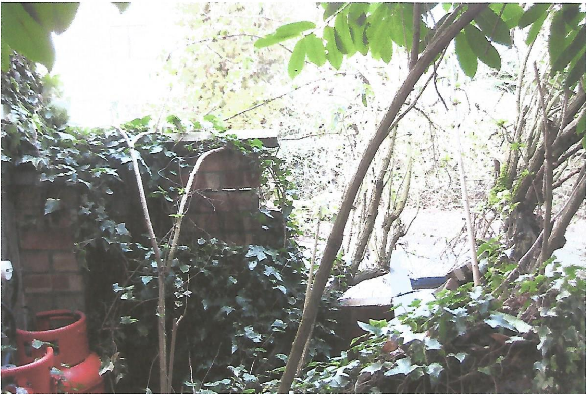
Picture 4 Damage to brickwall and lychgate looking from garden
