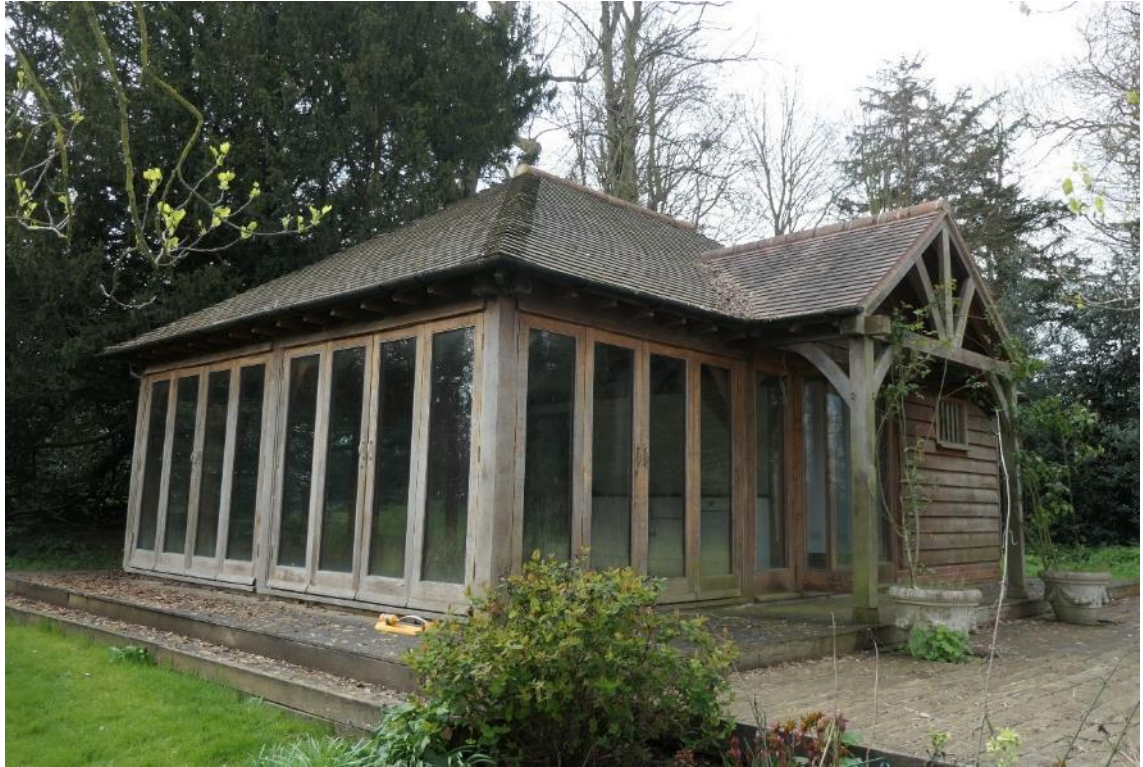
Photo 7 , north and east aspects of building one within survey area D, looking southwest.
