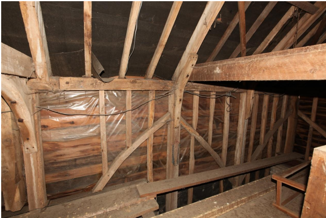
Illus. 28. The eastern interior of the barn's southern bays (1) showing the original knee-braces linking the principal rafters and storey posts with curved nailed primary braces in a style more usually associated with 18 th century pegged examples. The softwood tie-beam to the right is a 20 th century insertion and an original face-halved and bladed scarf joint is visible in the roof-plate to the left.
