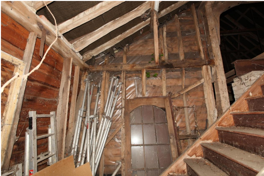
Illus. 20. The northern internal wall of the western lean-to porch (1), showing the narrow studs and diagonal primary brace of its original framing. The tie-beam is pegged and tenoned to the western roof-plate on the left and to the storey post of the barn's main span on the right.
