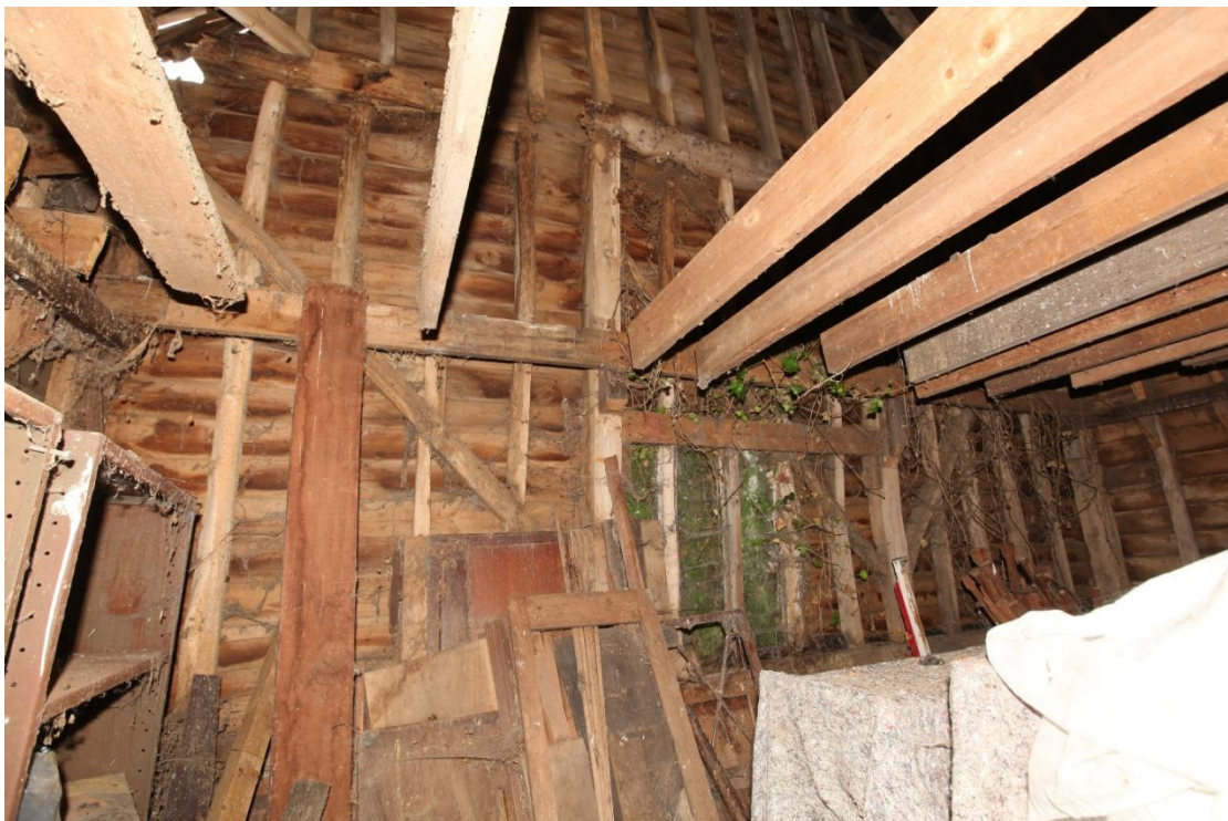
Illus. 16. The interior of the barn's northern gable (1) showing its 20 th century window and largely intact original framing with narrow-sectioned studs interrupted by nailed diagonal primary braces.
