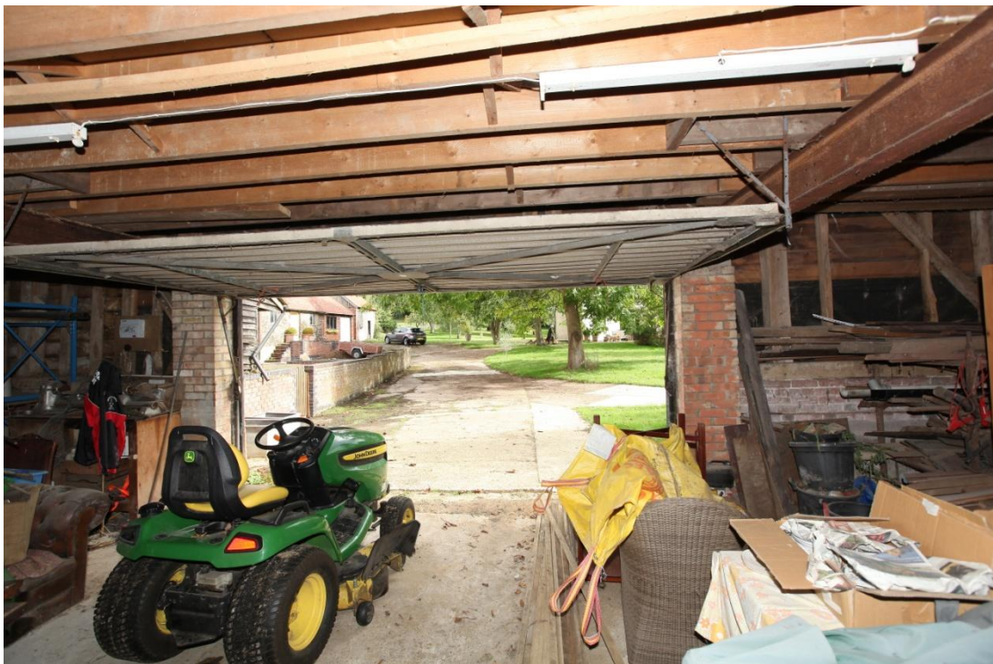
Illus. 14. The eastern interior of the barn (1) showing the modern 'up-and-over' garage-type door which replaced the original entrance in the central bay and extends into the adjoining bay to the right, cutting the storey post and door jamb in illustration 29.
