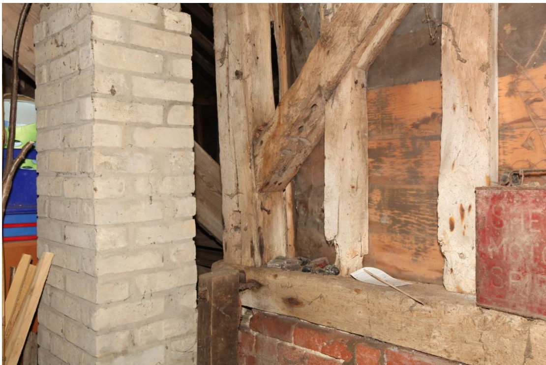
Illus. 12. A detail of the barn's rear (western) wall to the right in illustration 11 showing a modern brick pier supporting the loft and the empty mortices in both the storey post and the diagonal primary wall brace to the north of the porch which identify them as re-used timbers. The braces interrupt the studs and are nailed rather than tenoned at both ends.
