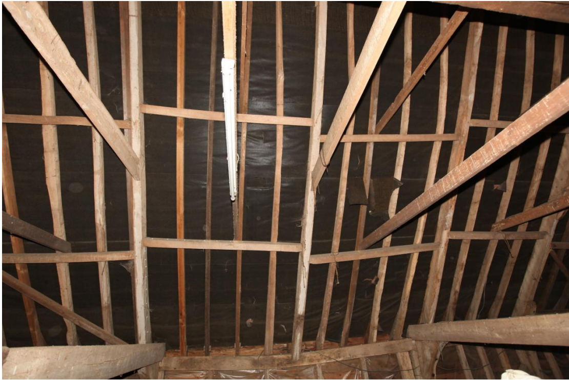
Illus. 33. The largely intact eastern roof structure above the central threshing bay (1) showing a small number of renewed softwood rafters and inserted nailed collars. The original timber consists of elm and oak. The upper collars of the three central principal trusses are pegged but not braced.
