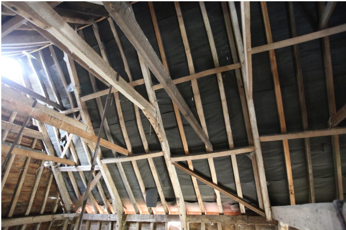
Figure 26. A detail of the largely original roof structure to the east of the northern bays (1). A small number of rafters have been renewed in light-coloured softwood and additional softwood collars inserted in the centres of each bay (lodged on the lower purlins and secured by vertical iron straps).
