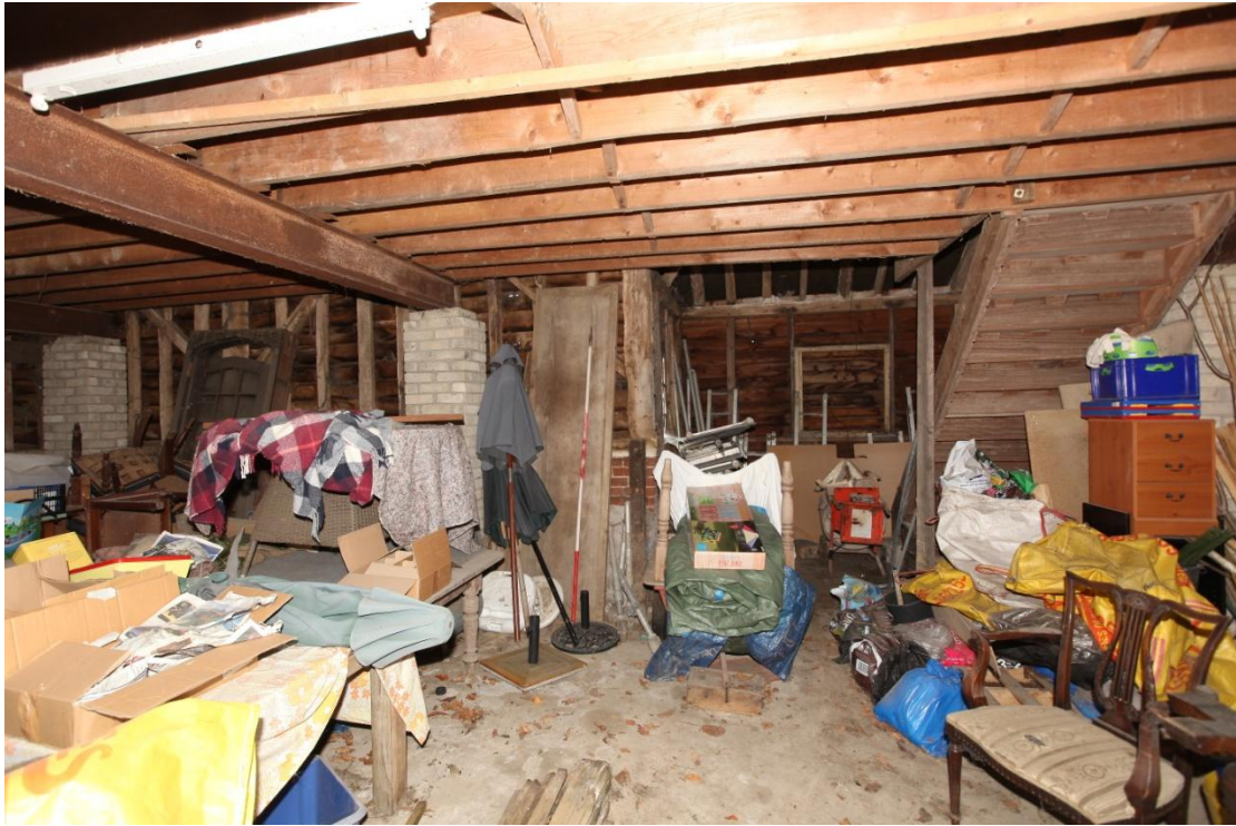
Illus. 13. The western interior of the barn (1) showing the modern loft stair in the central rear porch to the right and the brick piers supporting its RSJs in the southern bays to the left. The floor consists of 20 th century concrete with no trace of the boarded or brick threshing floor that would have occupied the central bay.
