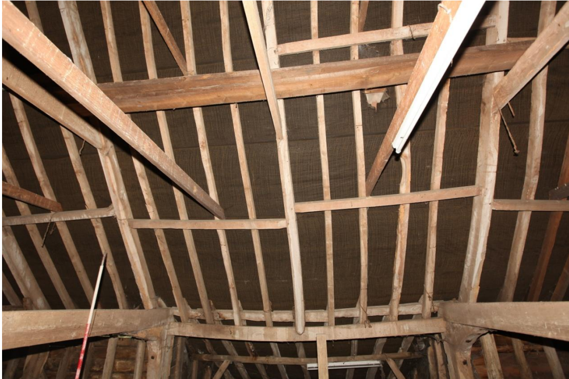
Illus. 35. The intact western roof structure above the rear lean-to porch showing the two arch-braced tie-beams flanking the central bay.
