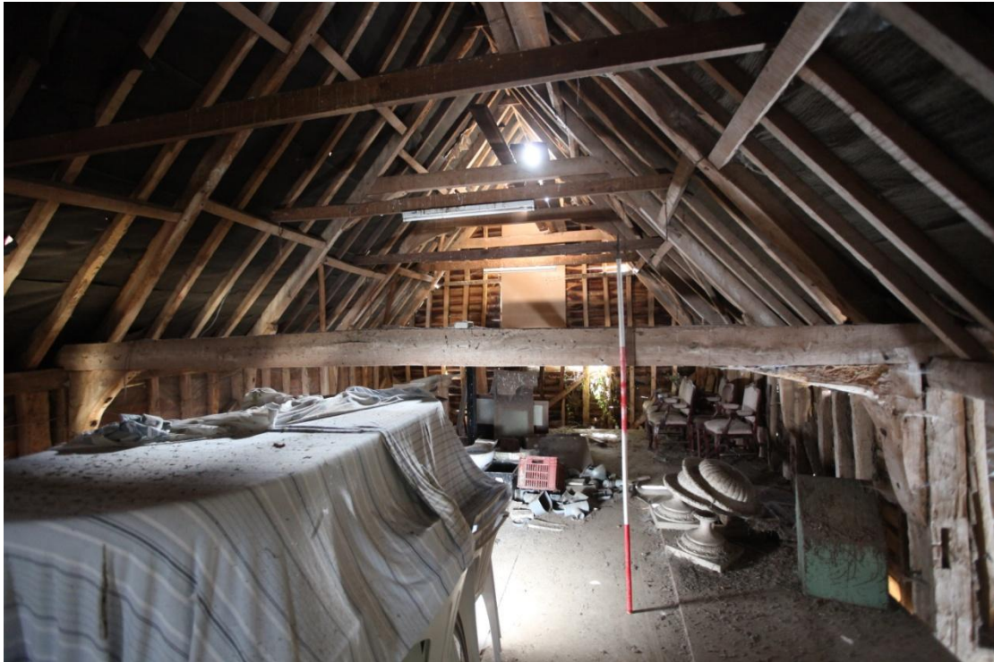
Illus. 27. The southern bays of the barn (1) seen from the central threshing bay with the latter's original knee-braced tie-beam in the foreground.
