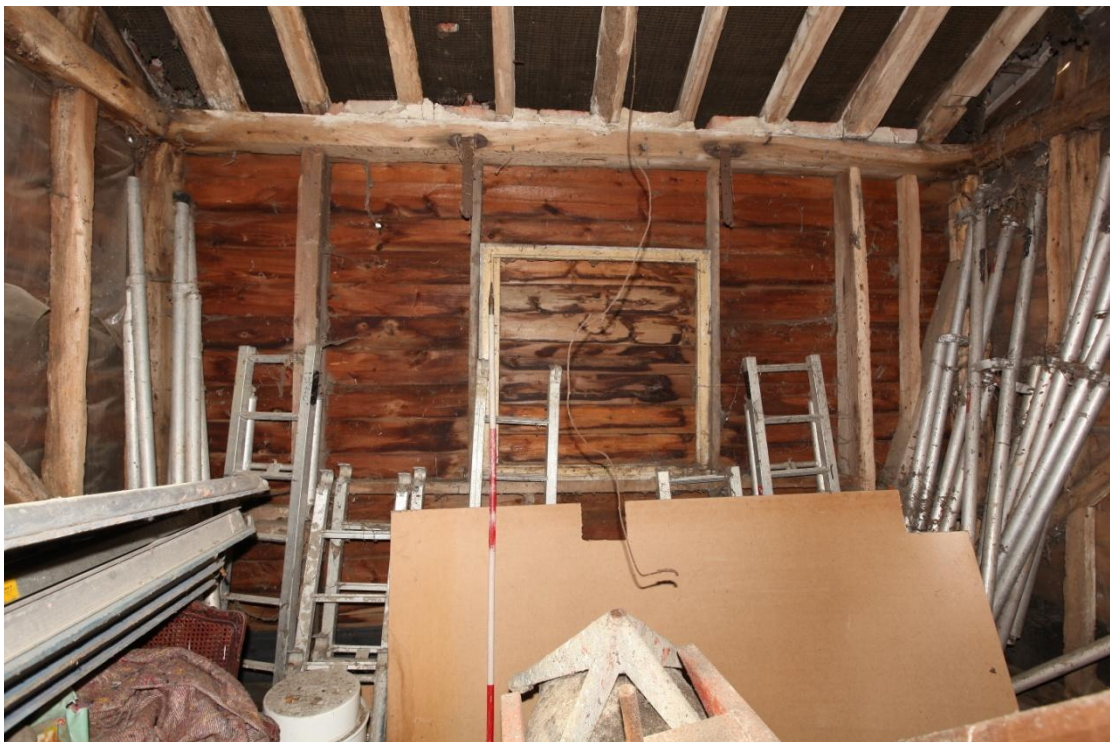
Illus. 18. The western interior of the rear lean-to porch (1) showing the original jamb of its doors pegged to the roof-plate on the right and a renewed softwood jamb in the original pegged mortice to the left. A mortice in the centre of the plate held the locking post of the doors and the iron hinges on each side evidently held a secondary vertically hinged hatch or shutter. The stud and diagonal brace to the right are also original.
