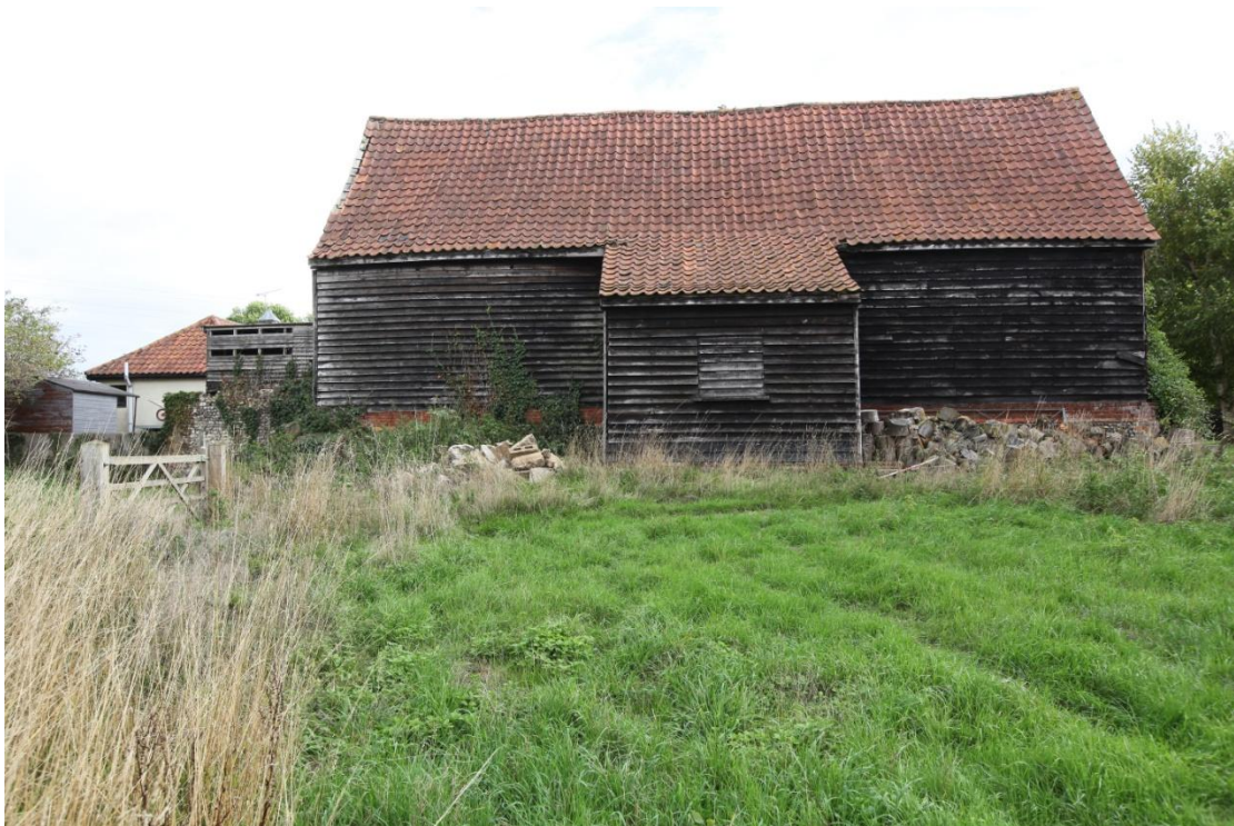
Illus. 8. The rear western elevation of the barn (1) showing the ostensibly original elm weatherboarding to the northern bays on the right which contrasts with the 20 th century external pine boarding elsewhere. The rear porch was built with 2.1 m or 7 ft wide doors that rose to its roof-plate but their position is blocked by the later cladding.
