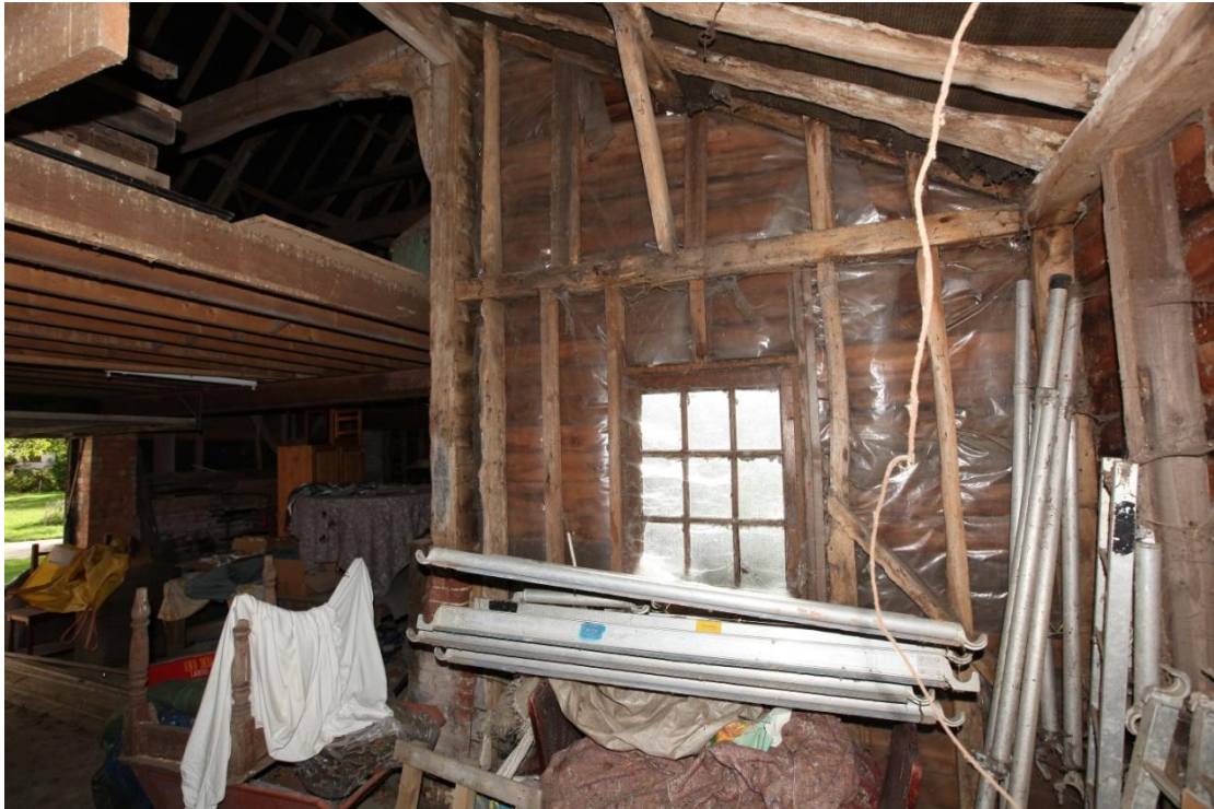
Illus. 21. The southern internal wall of the western lean-to porch (1), showing the narrow studs and diagonal primary brace of its original framing, partly cut by a later window. The tie-beam is pegged and tenoned to the western roof-plate on the right and to the storey post of the main span on the left.
