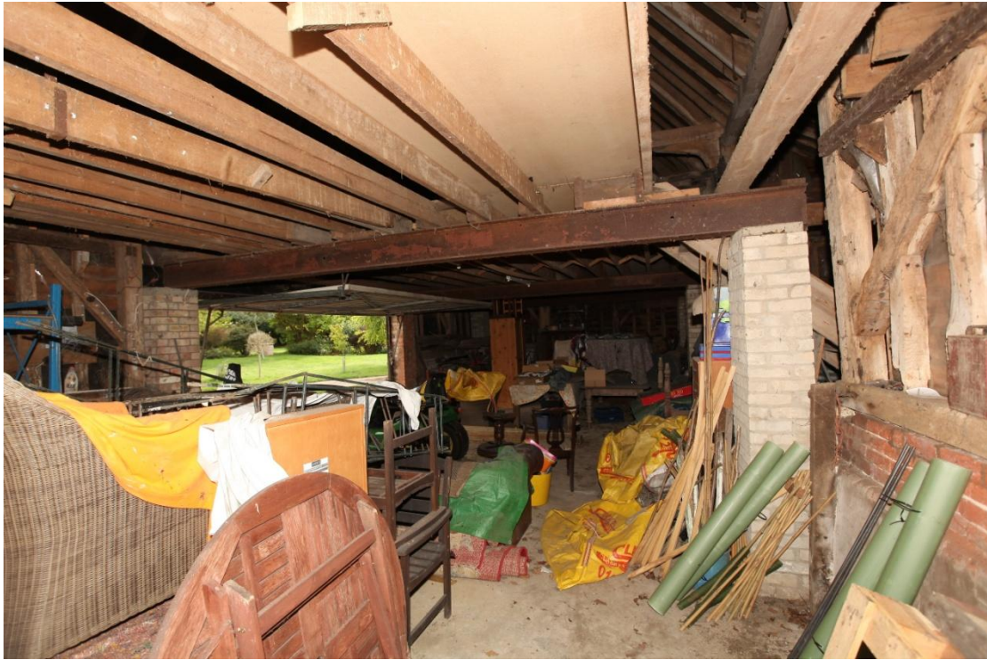
Illus. 11. A general view of the barn's interior (1) as seen from the north, with the 20 th century garage door in the eastern wall to the left. The barn contains a late-20 th century loft of narrow-sectioned softwood joists supported by RSJs on brick piers which conceals the roof structure from ground level.
