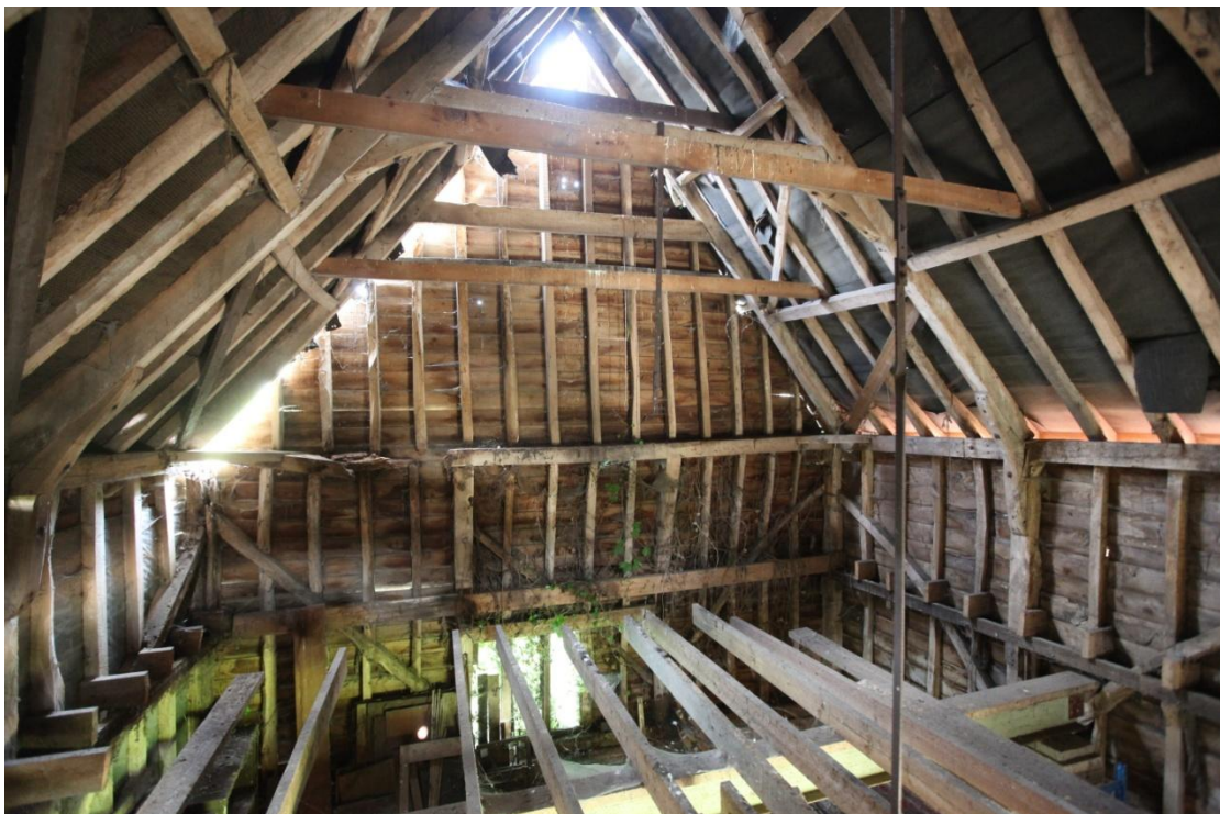
Figure 24. The northern internal gable of the barn (1) from the loft showing the original bolted knee-braces securing the two storey posts of the northern bays directly to the principal rafters in the absence of tie-beams (thereby increasing headroom). The steeply pitched roof structure consists of two tiers of staggered butt-purlins with knee-braces to the pegged collars and survives largely intact with evidence of some re-used material. Note the old break in the gable tie-beam to the left, apparently caused by water ingress.
