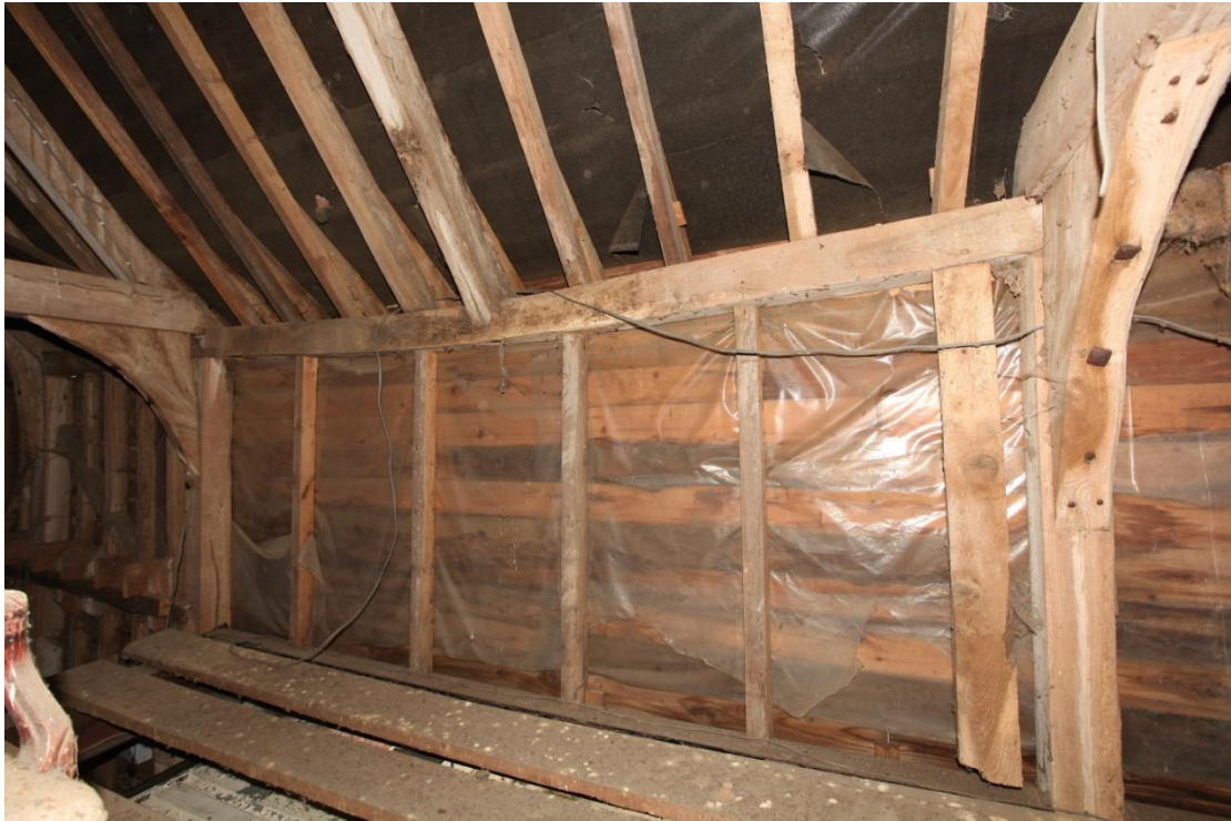
Illus. 29. The eastern roof-plate of the barn's central bay showing an original door jamb adjacent to the storey post on the right, pegged and tenoned to the plate. An empty pegged mortice for an identical jamb is visible to the left of the plate with an unpegged mortice for the locking post in the centre. The present wall studs are modern and lie above the garage door that cuts the post to the right and has caused the plate to bend beneath the central roof truss.
