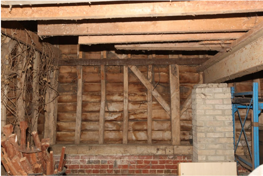
Illus. 17. A detail of the eastern interior of the barn's northernmost bay (1) showing its ostensibly original elm weatherboarding and narrow-sectioned studs interrupted by a diagonal primary brace in the typical 19 th century manner. The rail and truncated joists of an earlier inserted loft are visible above the RSJ.
