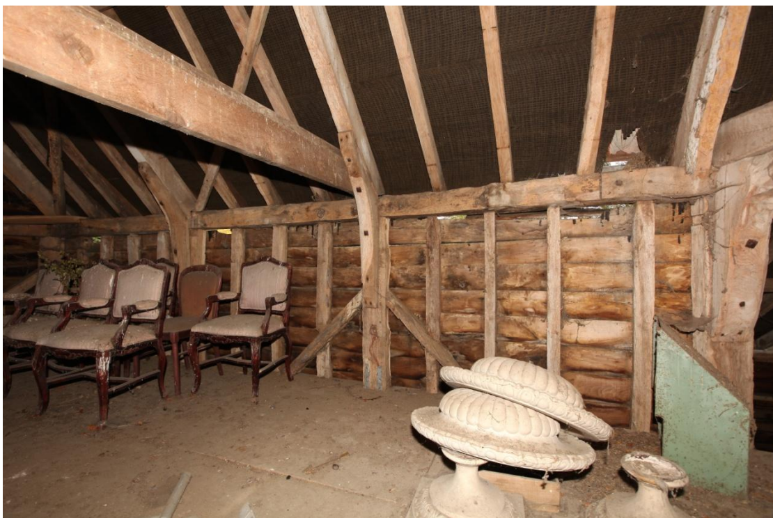
Illus. 30. The western interior of the barn's southern bays (1) showing their intact original framing and rafter knee-braces with the original elm weatherboarding. A face-halved and bladed scarf joint of typical post-medieval form is visible to the right.
