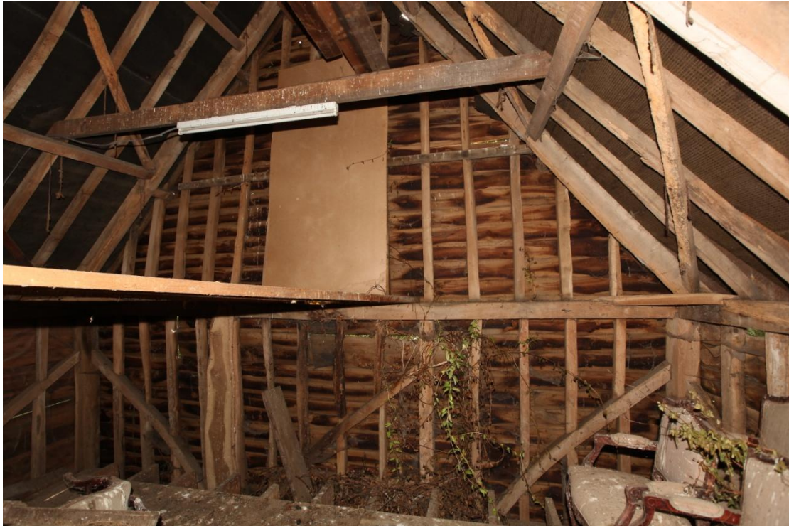
Illus. 31. The southern internal gable of the barn above the loft showing its intact asymmetrical framing with two curved braced descending from the right and one to the left. Unlike the tie-beams of the threshing bay which are dovetailed to the roof-plates those of both gables are tenoned at the same level with their junctions strengthened by diagonal tie-beams as shown in illustration 32. The boarding above the gable tie-beam blocks a 20 th century inserted window and there is no obvious evidence of original vents.
