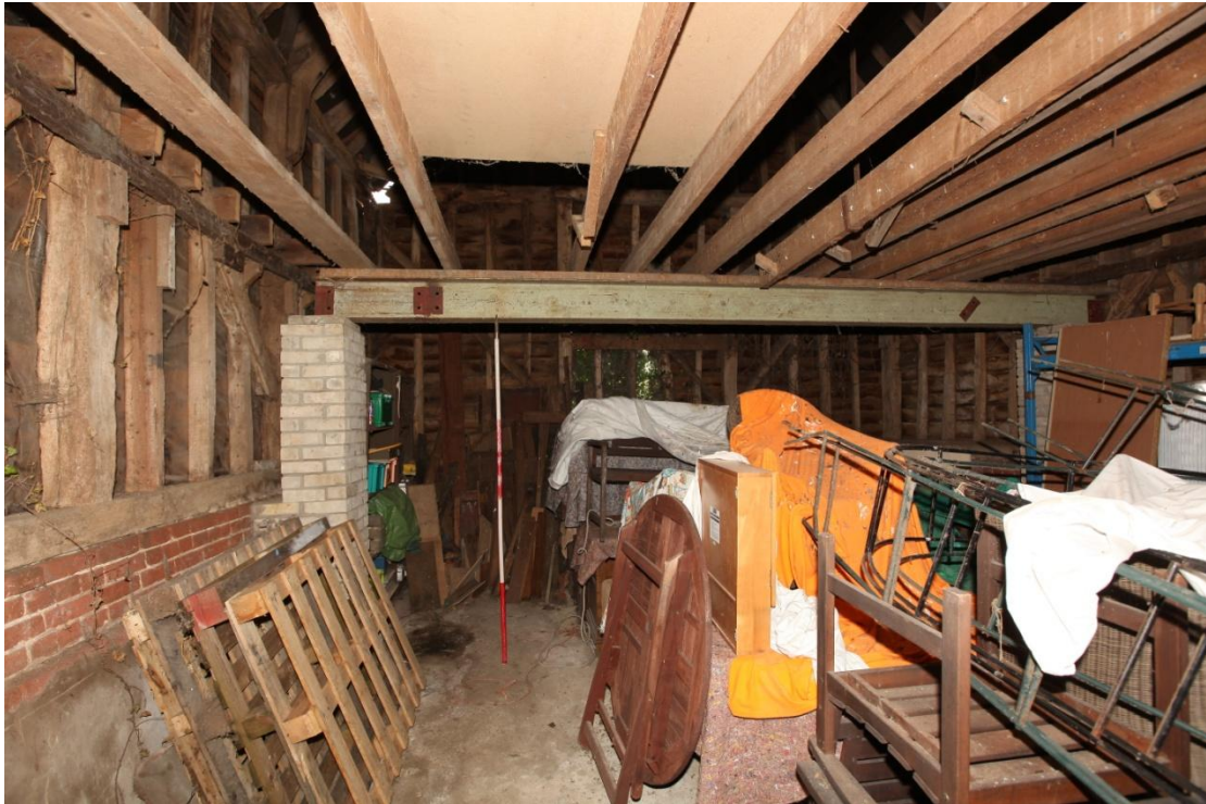
Illus. 15. The interior from the south of the northern bays of the barn (1) showing the late-20 th century loft from which a number of joists have been removed. The truncated joists and wooden supporting rail of an earlier 20 th century loft which the present structure replaced are visible on the western wall to the left.
