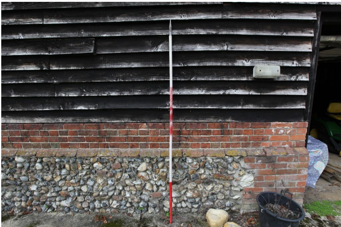
Illus. 6. A detail of the tarred 20 th century softwood weatherboarding to the barn’s eastern exterior (1) showing its original brick and flint-rubble plinth with modern brickwork to the jamb of the enlarged entrance on the right.
