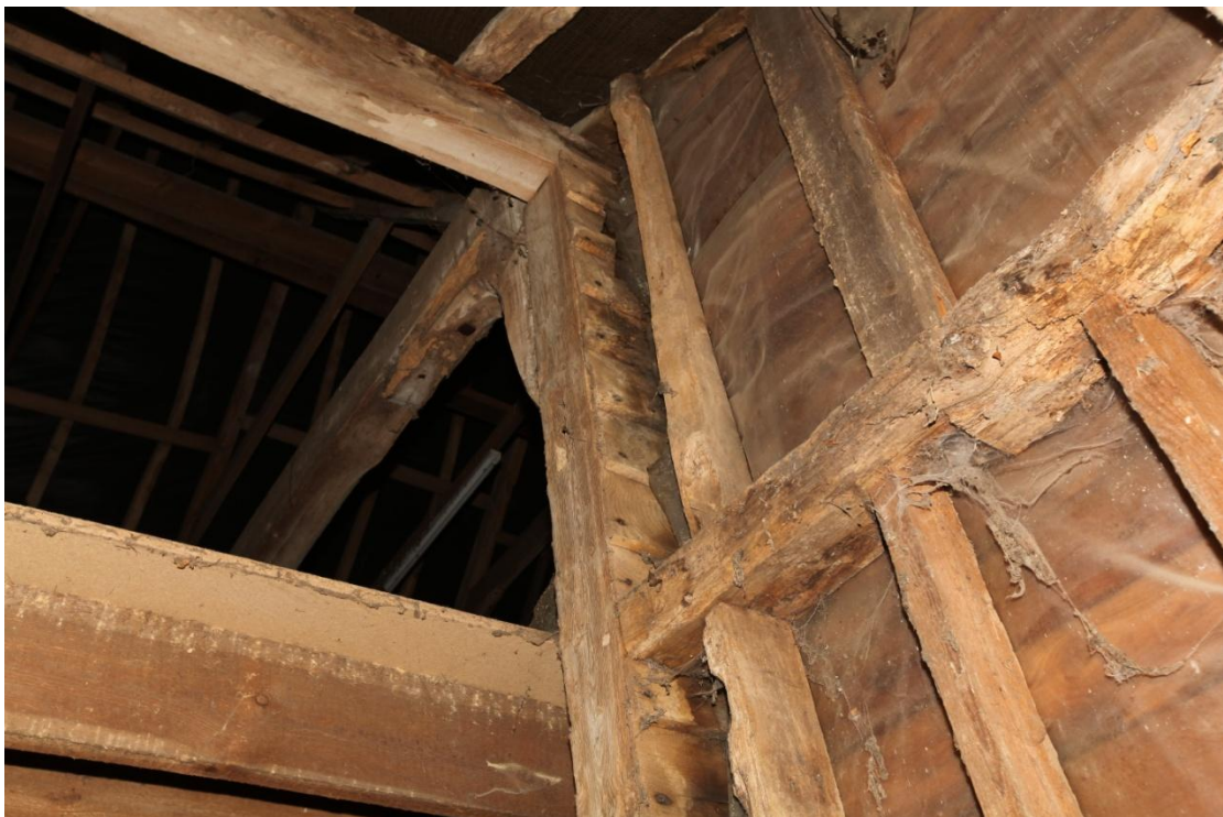
Illus. 22. A detail of the southern internal wall of the porch in illustration 21 showing its junction with the storey post of the main span (1). The horizontal tie-beam is pegged to the post and respected by the ends of the original elm weatherboards which continue externally but were protected by the porch from the application of tar. The adjoining roof-plate of the main structure at top left is devoid of mortices for studs or doors.
