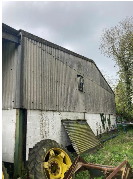
Fig 4 – North Elevation – Rear gable end of existing barn, viewed from northern boundary.
