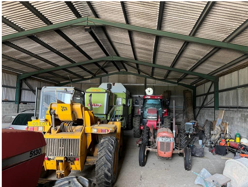
Fig 5 – Internal view of North gable, showing roof structure and supporting portal frames.
