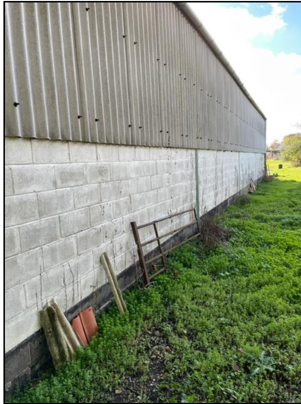
Figure 7: View along western frontage of site showing no flood pathways into building
