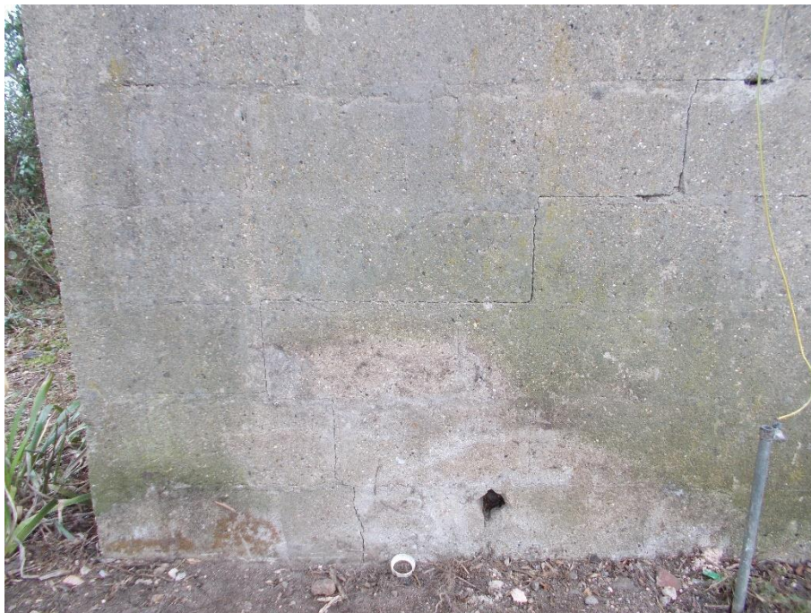
Photograph 6: Minor cracking to west elevation blockwork
