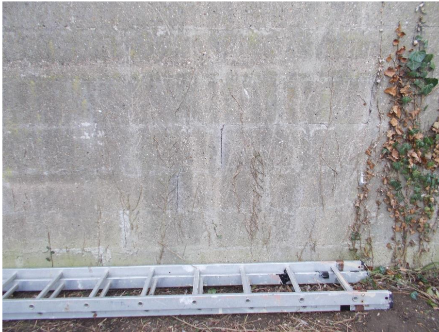
Photograph 5: Minor cracking to north blockwork
