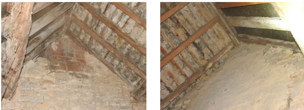
Figs. 21 & 22 Cobwebbed gable ends
