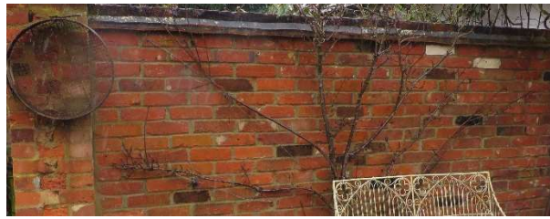
Brick for brick plinth and extension wall to match those used in existing garden wall.
