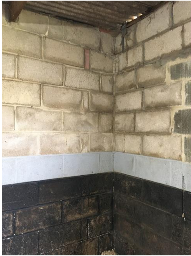
Photograph 7 Stables – Cracking internally
