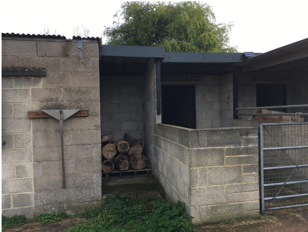
Photograph 5 Stables – External cracking at top RHS corner
