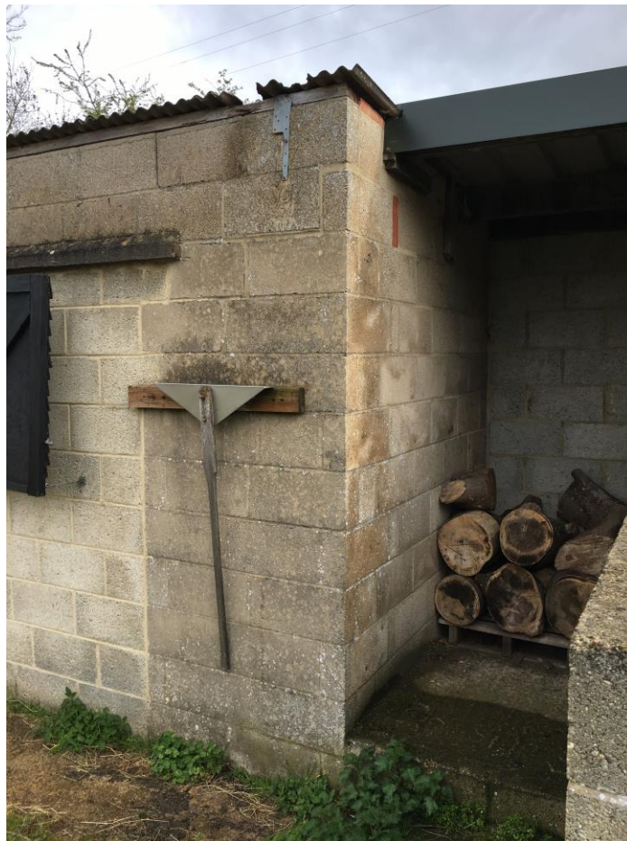
Photograph 6 Stables – External cracking and discontinuity of roof
